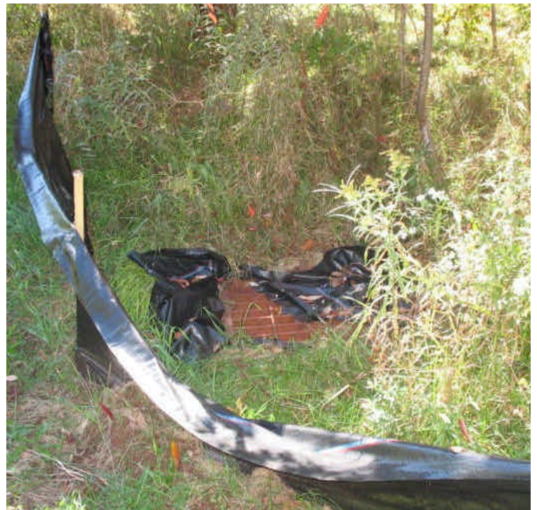
Catch Basin protection off Stony Brook Rd.
