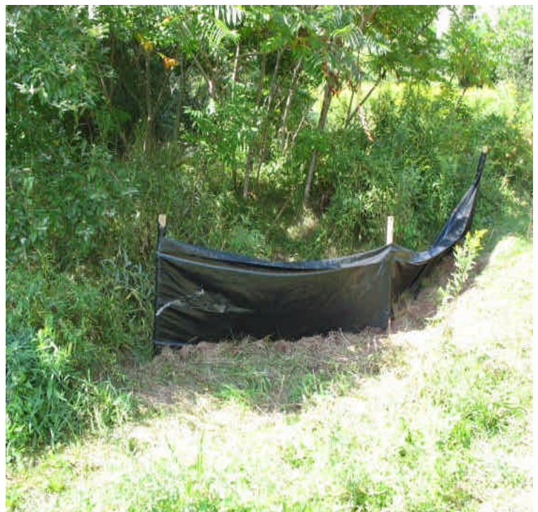
Silt fence and silt liner at catch basin inlet off Stony Brook Rd.
