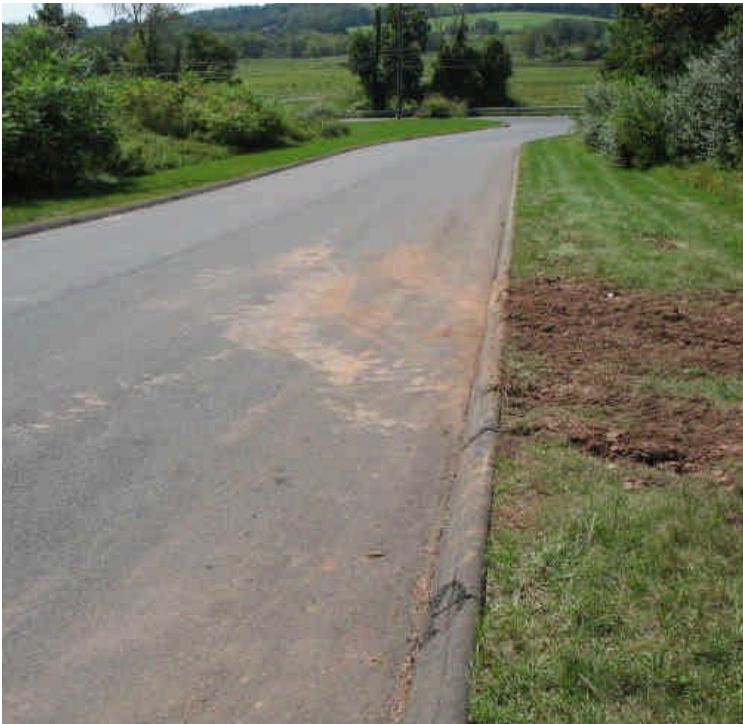
Sweep sediment from the construction entrance off Stony Brook Rd. Continue to watch this area for tracking
