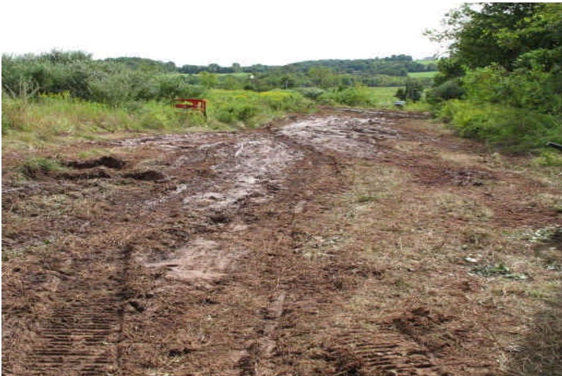
New site entrance located adjacent to Stony Brook Rd. Entrance will be left to revegetate and an existing roadway will be rebuilt along the wetland once permits are obtained.
