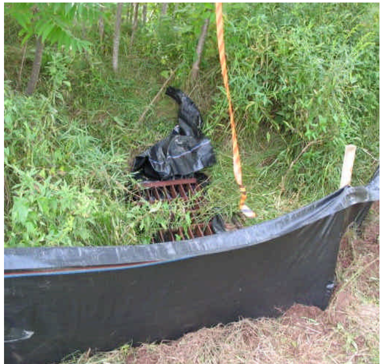
Silt fence and silt liner at catch basin inlet off Stony Brook Rd.
