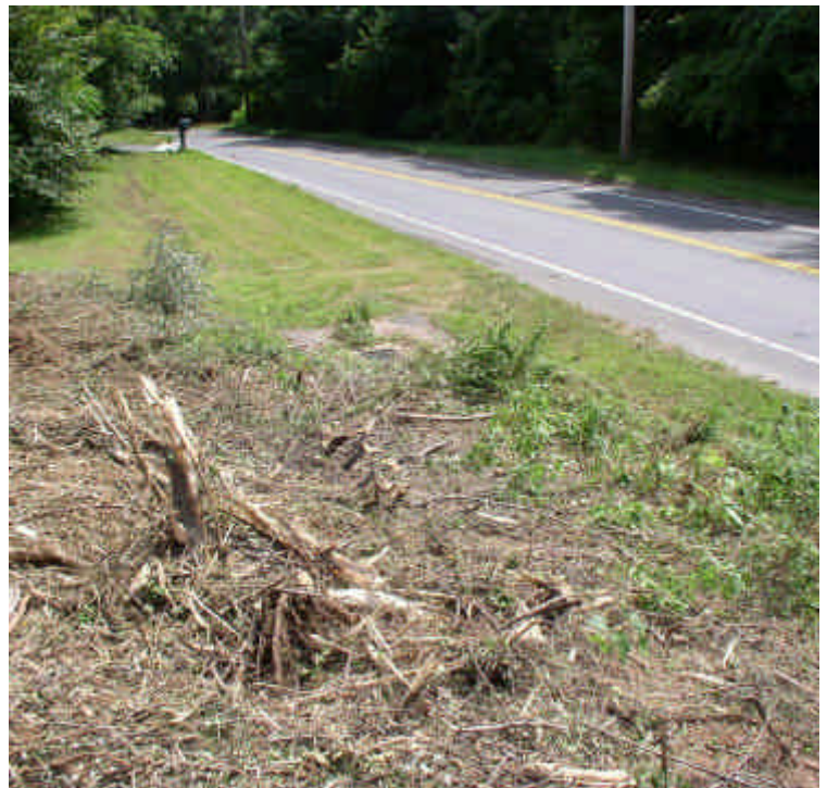
Haybales are needed around the catch basin along Route 68.
