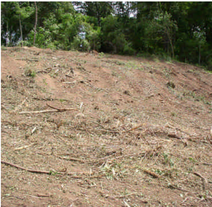
Steep, exposed slope needs water bars and/or other erosion controls. Retain as much vegetation as possible to reduce disturbed sediment.
