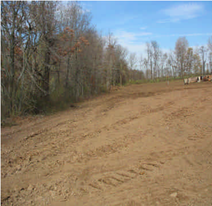
Silt fence installation needed above drainage ditch at the contractor receiving yard & staging area.
