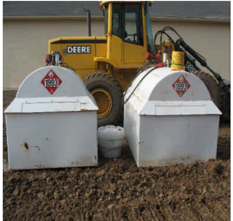
Fuel tanks were empty, nozzles turned up, and a spill kit was added the contractor yard until further containment can be constructed.
