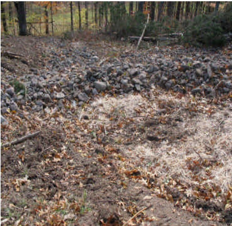
Mulch, check dam, and riprap installed at the end of the access road off Black Walnut Dr.
