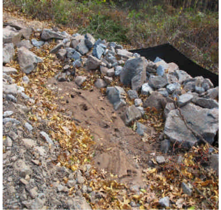
Sediment captured at the riprap sediment trap from the recently installed culvert/swale along Black Walnut Dr.
