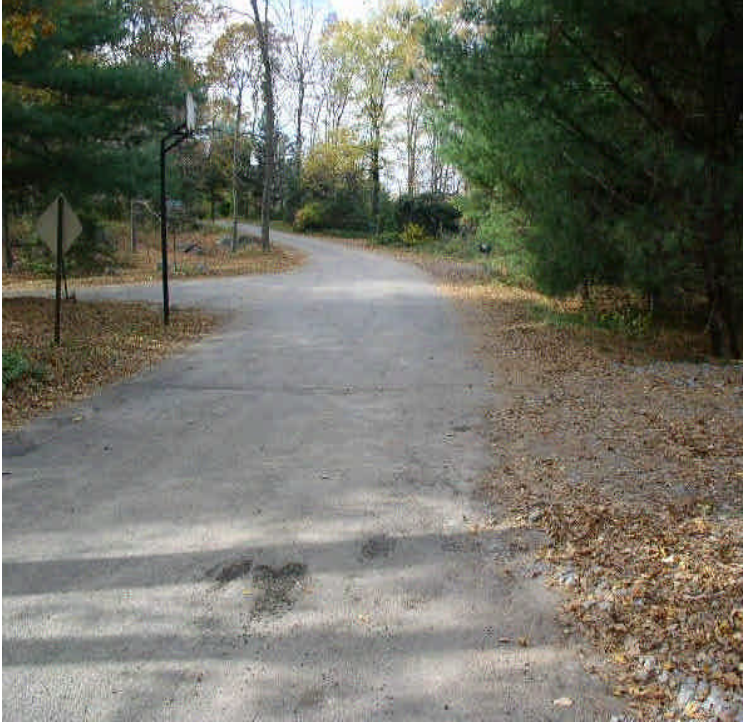
Tracking was not noted on Oxbow Road; the roadway was cleared of sediment.
