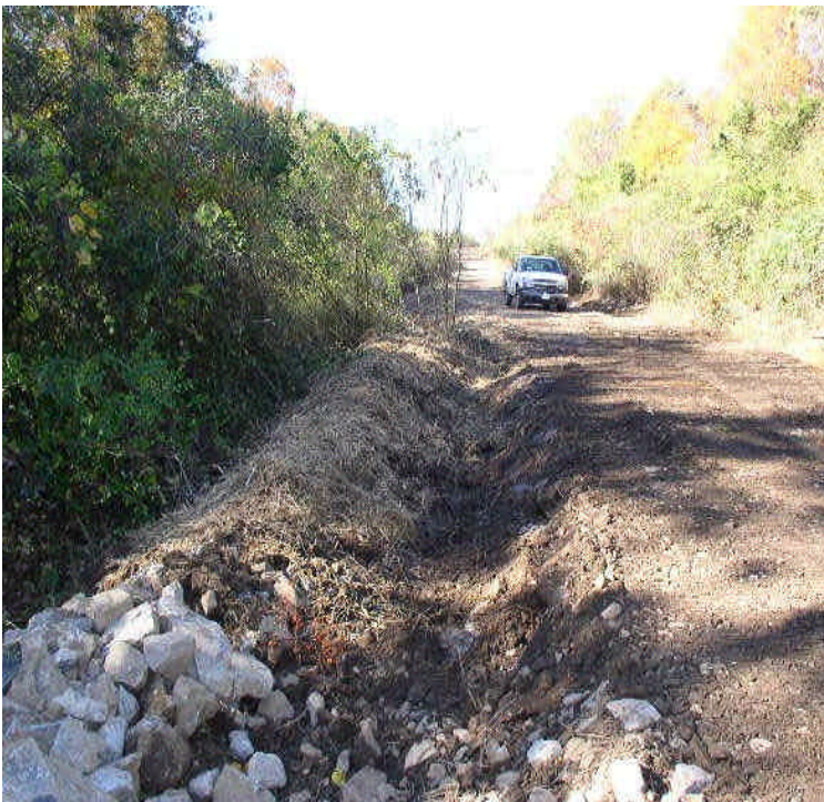
Completed access road off Black Walnut Dr with stormwater controls in place. A swale was installed and road slopes were temporarily stabilized with mulch.
