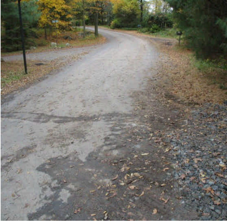
Minor mud and sediment tracking observed on Oxbow Road.
