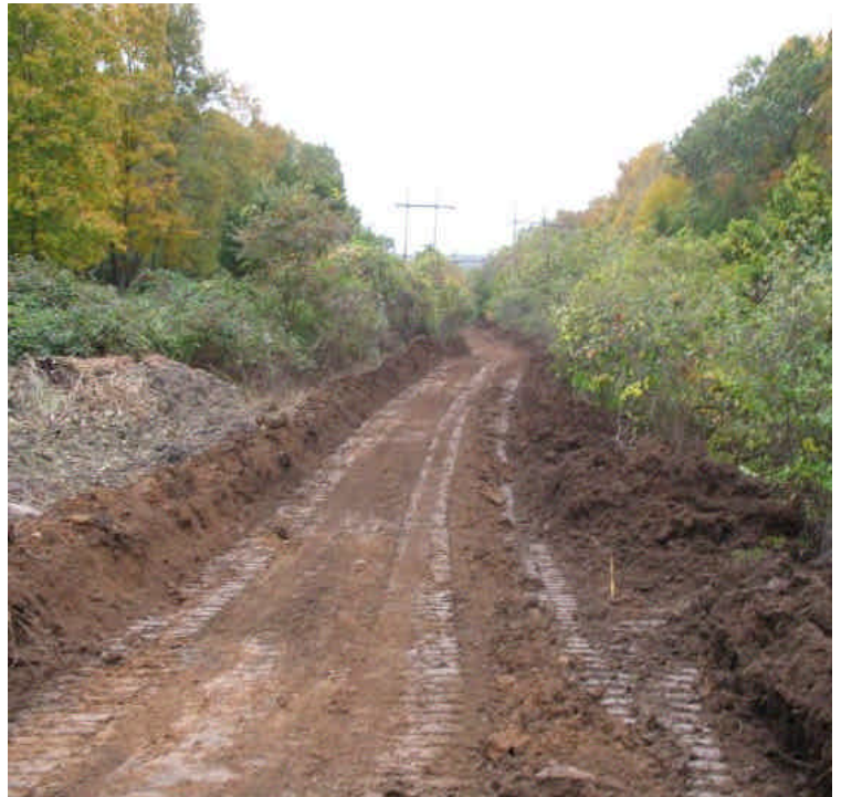
Access road construction within the ROW off Black Walnut Dr. Work remains outside of all wetland buffers.
