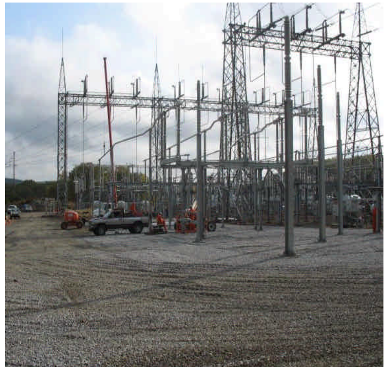
New foundations installed, these portions of the site are graded and stabilized.
