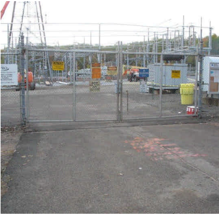
Site entrance, no new equipment spills or leaks, spill kits are onsite.
