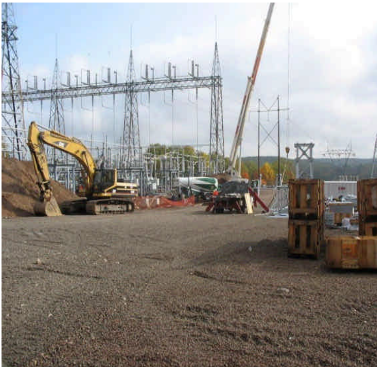
New excavations for foundations; stockpiles are internal to the yard and remain contained.
