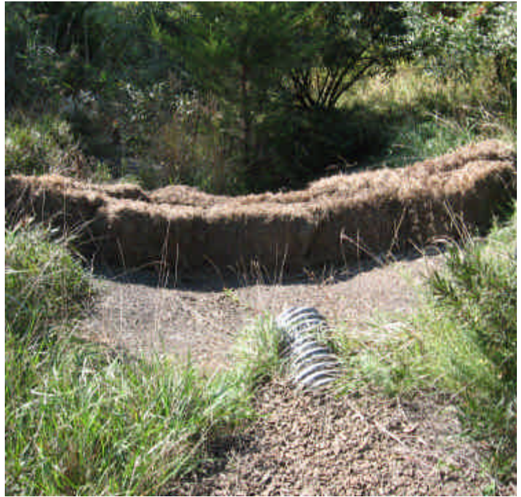
Drain outlet controls remains secure.
