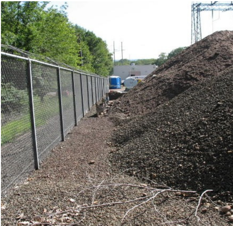
Silt fence located around the soil stockpile in the northwestern corner of the site looks good, soils contained.
