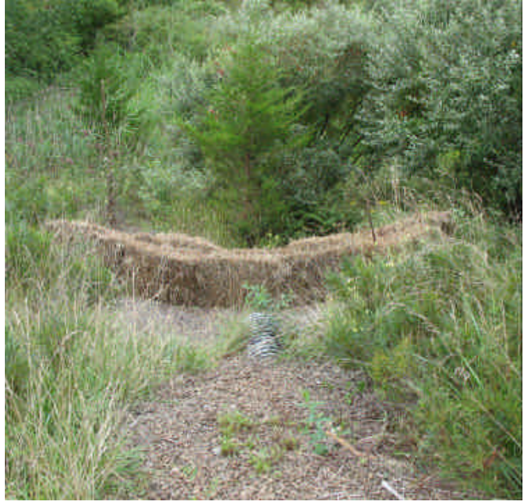
Storm water outlet pipe upgradient of the wetland, on the south side of the site. Controls are in place.
