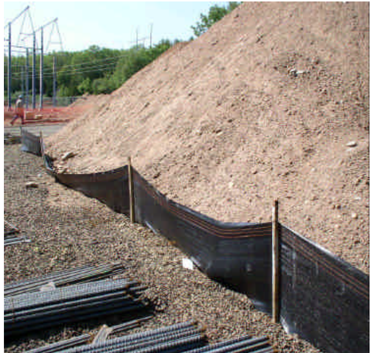
Silt fence added along stockpile at the northeast side of site; repair the section that came down and monitor. The section in disrepair is located well within the site.
