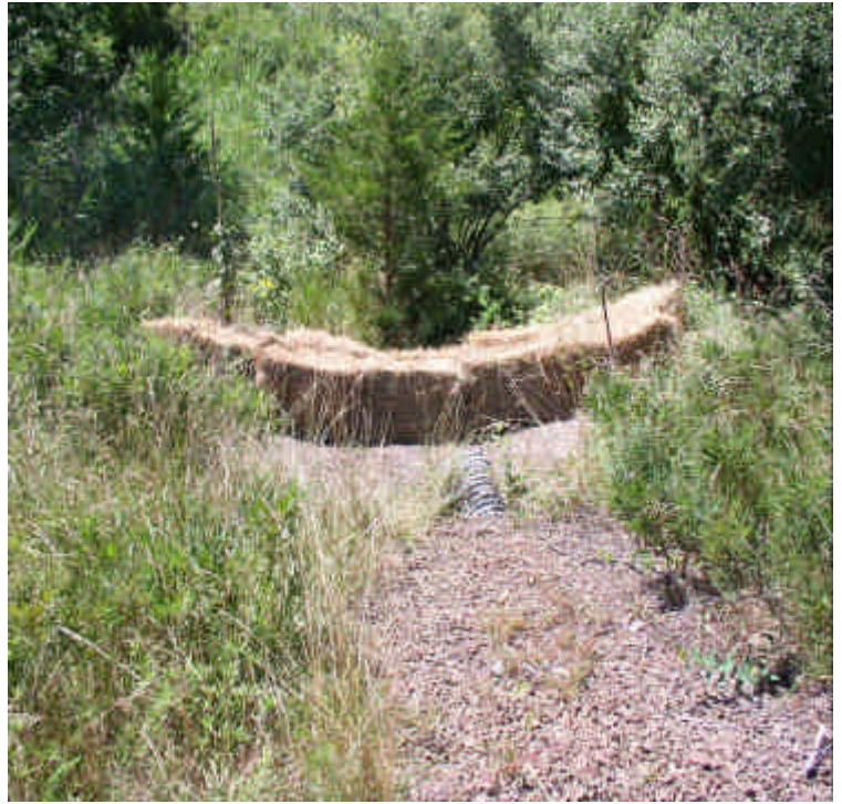
Storm water outfall pipe upgradient of wetland, south side of the site. Haybales were installed.
