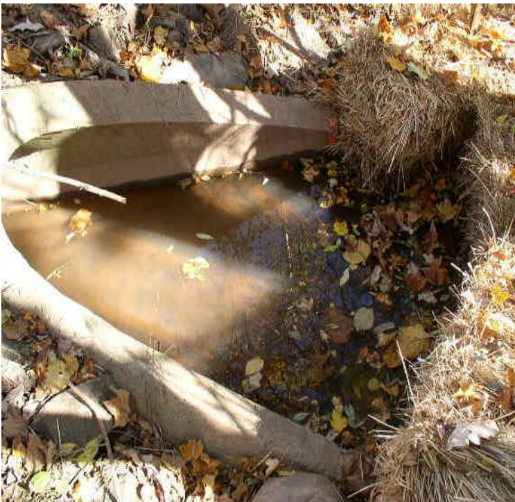
Sediment continues to settle out in the bottom of the storm drain outlet. New haybales have been installed.
