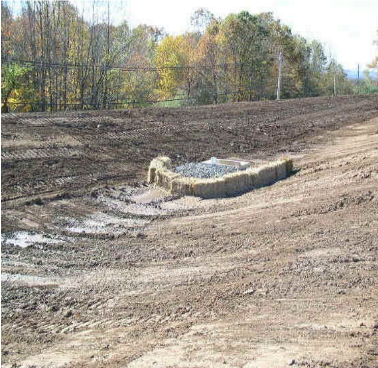
Final grading and installation of detention basins above the retaining walls along Carpenter Lane. Controls were in place at the inlets.
