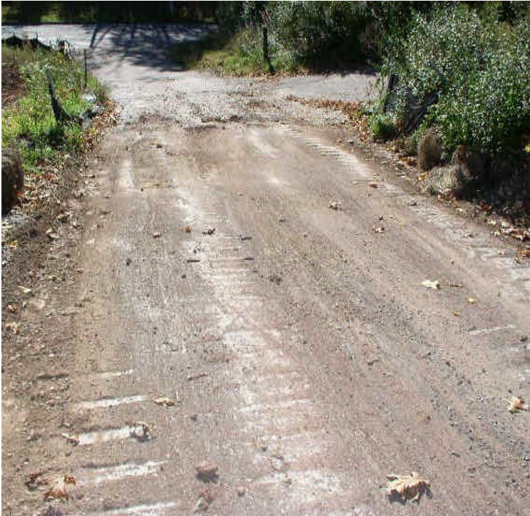
Old Zolnik property entrance at Carpenter Lane. Haybales need to be placed across the driveway.
