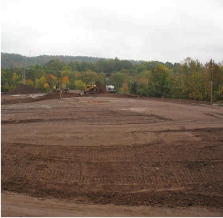
Final grading and installation of detention basins above the new retaining walls along Carpenter Lane.
