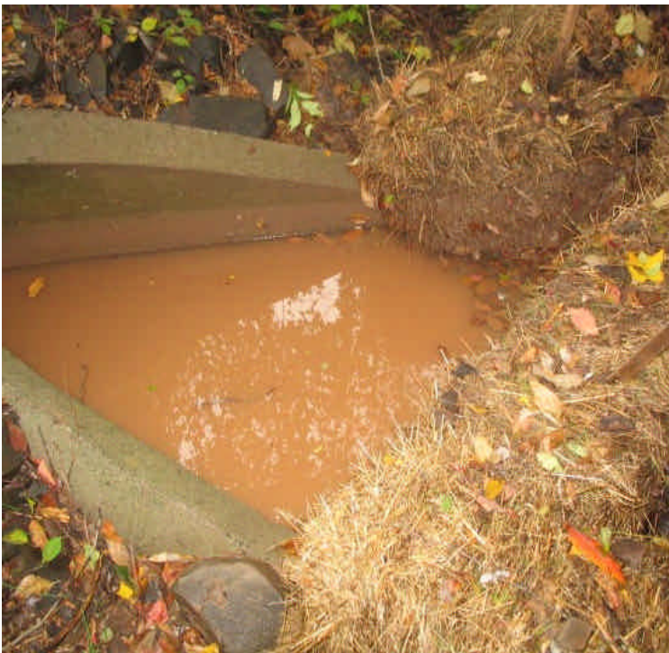
Turbid water continues to be present in the storm drain outlet.
