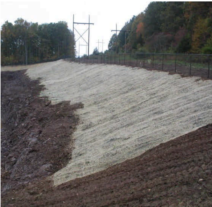
Erosion control mats were placed along the northern slopes. New perimeter fence is also installed.
