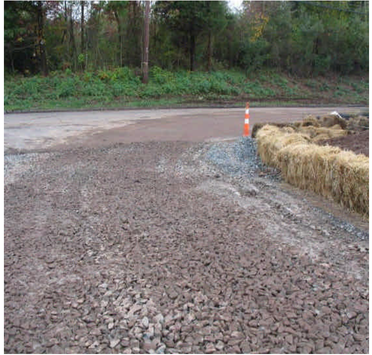
Carpenter Lane has observable sediment tracking and the roadway should be swept regularly. The entrance pad should be cleaned and improved. This is planned in the near future.
