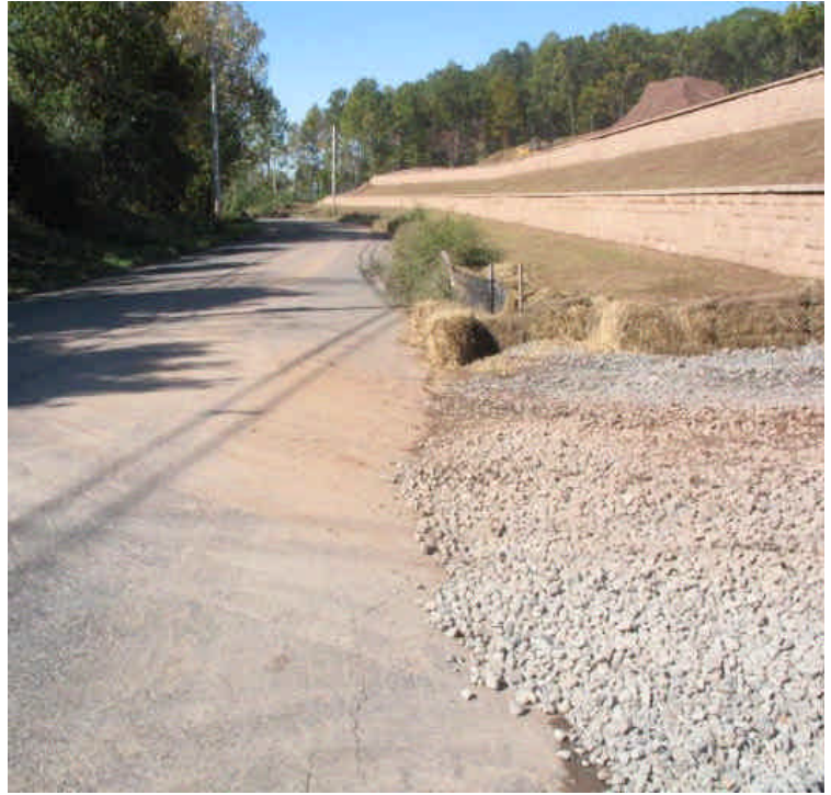
Carpenter Lane has some sediment tracking but is being swept regularly. New grass growth was noted on southern slopes.
