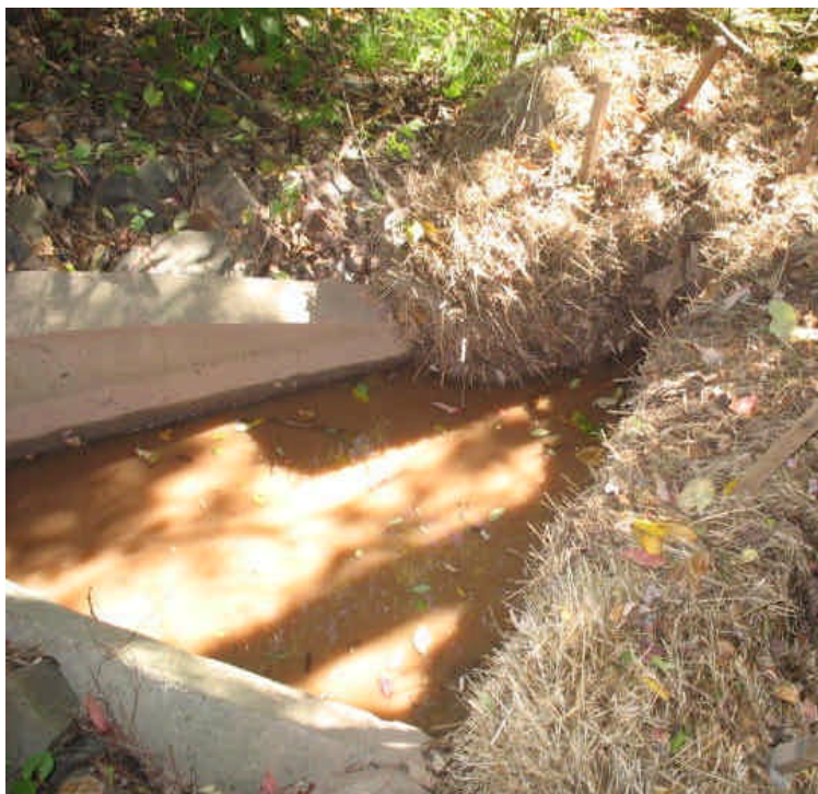
Turbid water continues to be present in the storm drain outlet.
