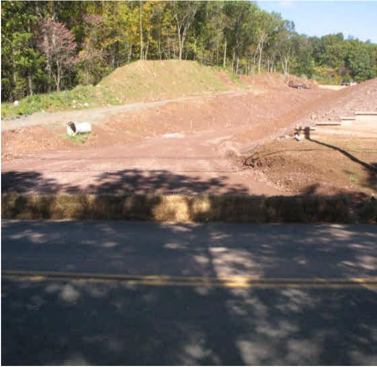
New, permanent site entrance installed on west side, with haybale barrier in place along Carpenter Lane.
