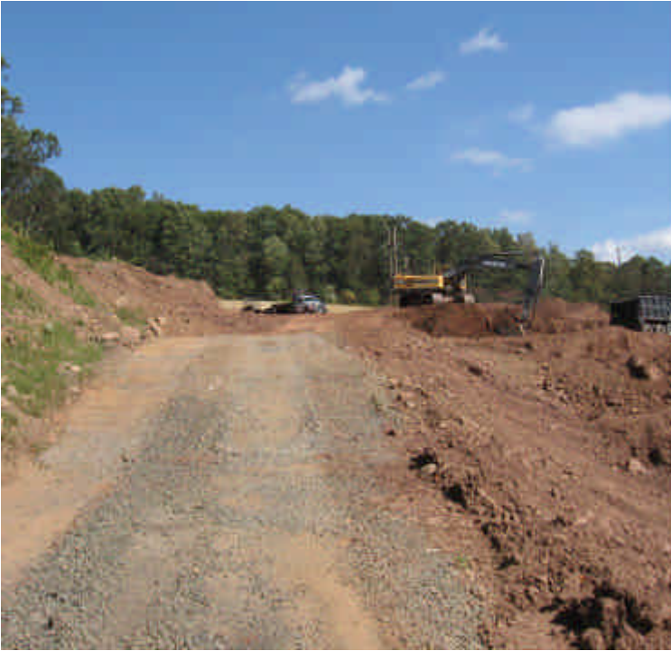
Driveway on western side of site is being used as truck entrance, not for exit; erosion controls remain functional.
