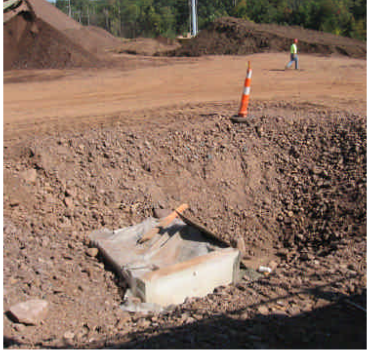
Stormwater inlet in southeast corner under construction but some controls are in place.
