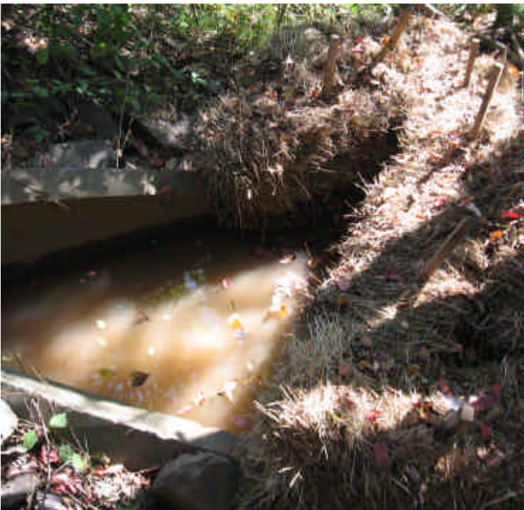
Turbid water in outlet remaining from the temporary storm drain system.
