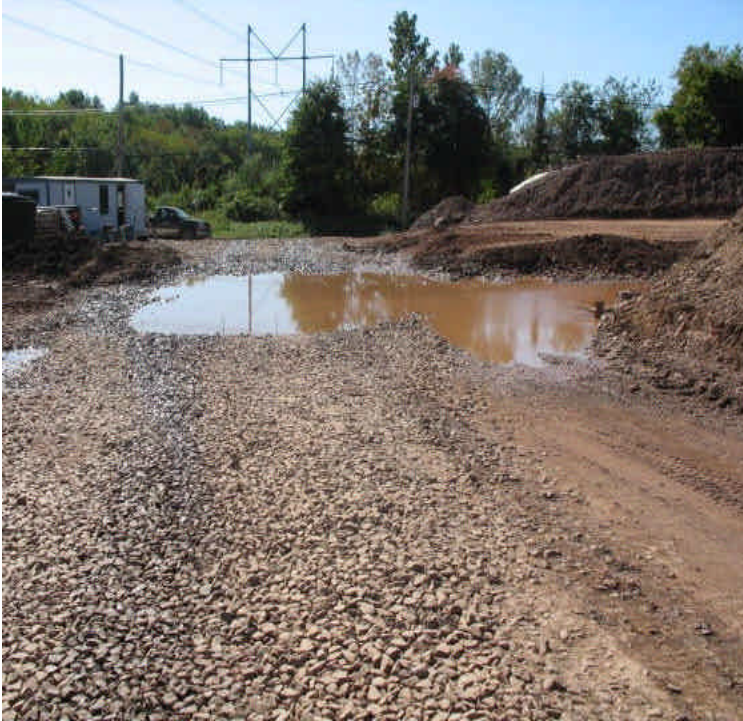
Crushed stone construction entrance pad with wheel wash area, Carpenter Lane should continue to be cleaned and swept, including the gutters, by hand if necessary.
