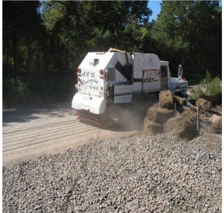
Street Sweeping along Carpenter Lane. More water is needed to reduce dust production.
