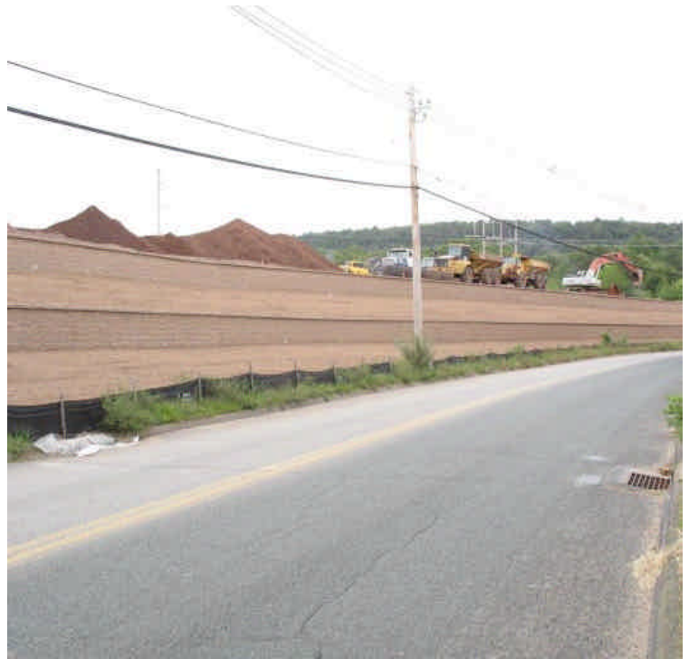
Loamed & fertilized area adjacent to the finished retaining walls should be seeded soon.
