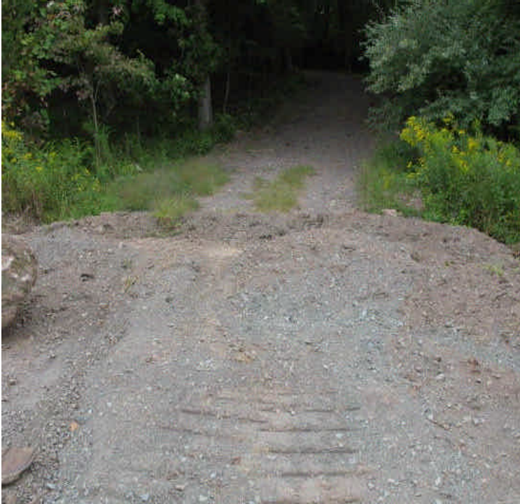
New water bar across old Zolnik driveway at the tree line northwest corner of the site.
