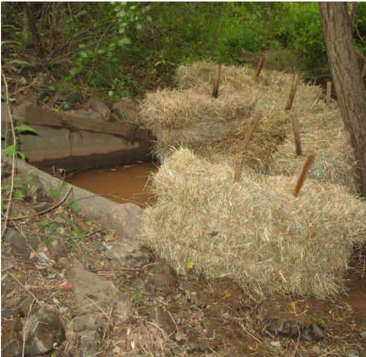
Sediment-laden water being flushed from the storm drain system and filtered before entering wetlands. Water pumping has been reduced. New haybales were added and sediment was removed from the outlet.
