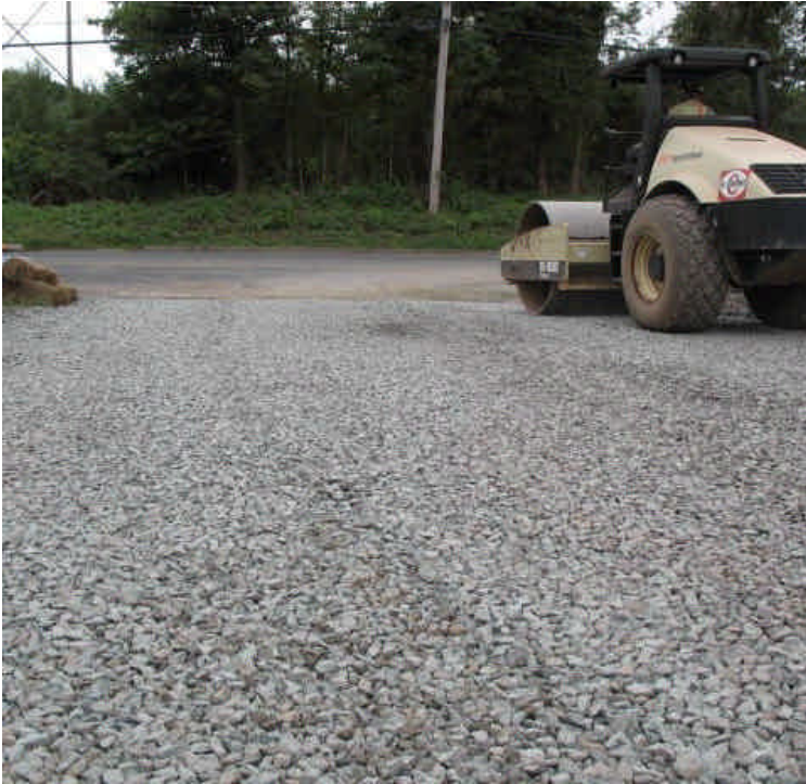
Crushed stone construction entrance pad refreshed with new stone, being compacted. Carpenter Lane should continue to be cleaned and swept, including the gutters, by hand if necessary.
