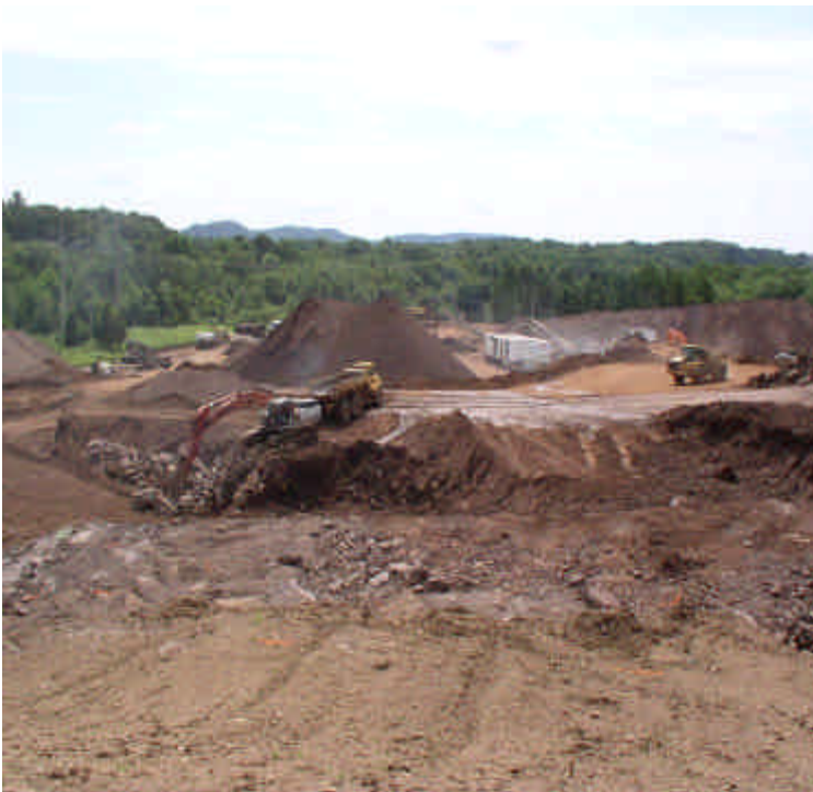
Major grading operations looking from northwest to southeast. Some airborne dust is noted. Continue to wet the soils when necessary.
