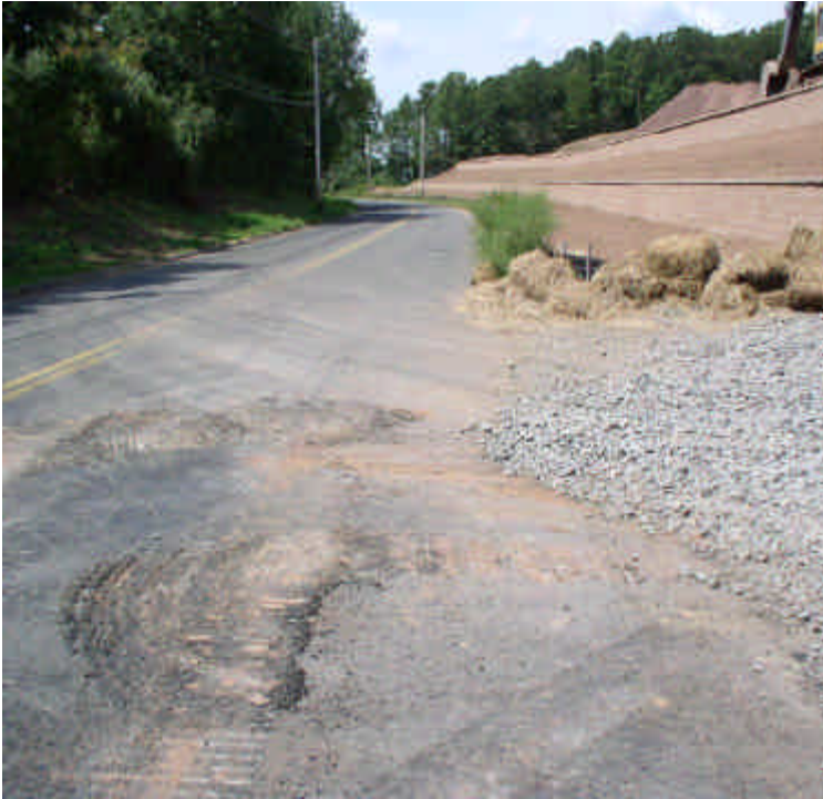
Crushed stone construction entrance pad is mostly clean; some minor tracking and road damage was noted on Carpenter Lane. The road should continue to be cleaned and swept, including the gutters, by hand if necessary.
