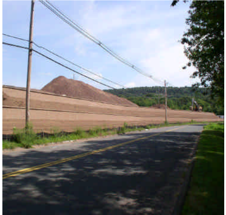
Final grading of loam is complete along the retaining walls and adjacent to Carpenter Lane.
