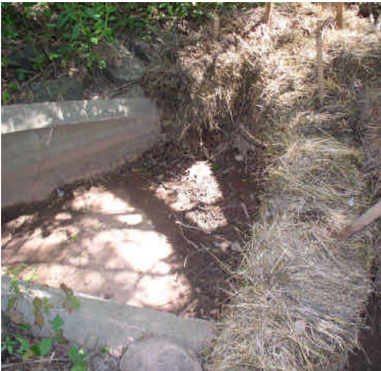
Sediment and old haybales have been removed from the end of the outfall pipe. Sediment removal should continue on a regular basis.
