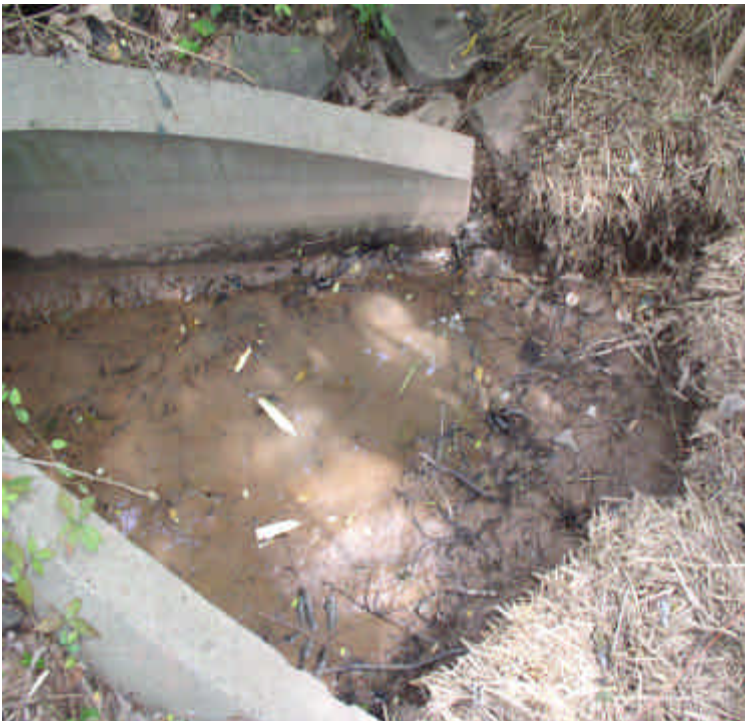
Remove accumulated sediment from the end of the outfall pipe on a regular basis.
