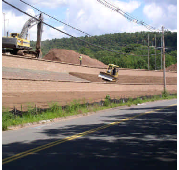
Final grading of loam is underway along the retaining walls and adjacent to Carpenter Lane.
