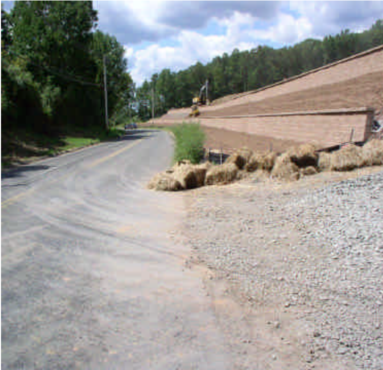
Crushed stone construction entrance pad is mostly clean; some minor tracking was noted on Carpenter Lane. The road should continue to be cleaned and swept, including the gutters, by hand if necessary.
