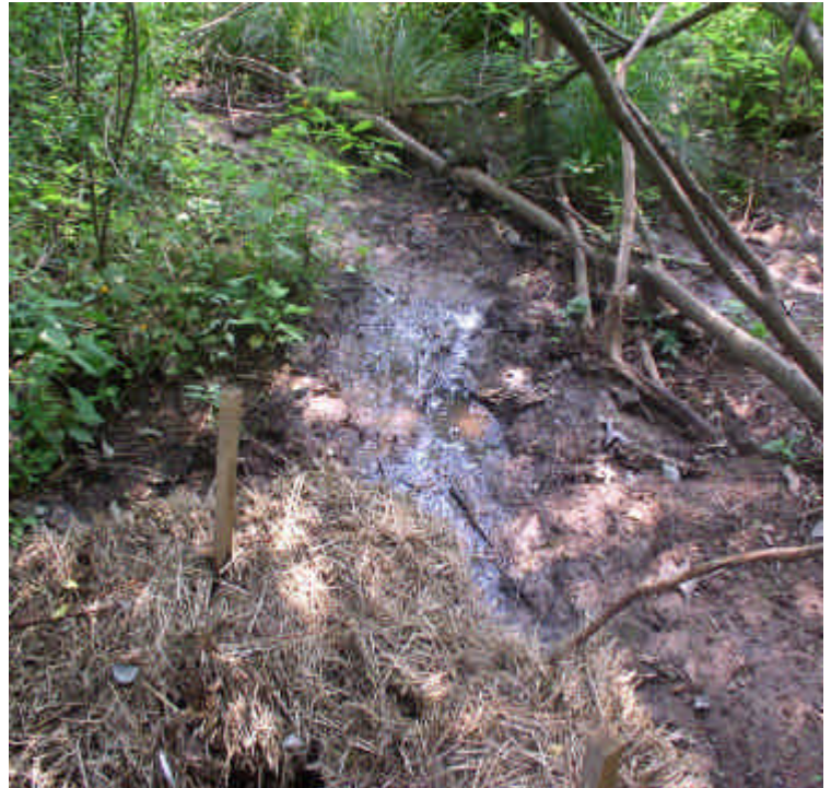
Flow from the culvert is being filtered by haybales prior to entering the wetland. Sediment accumulation from the previous rain events will be removed when standing water in wetland has dried.
