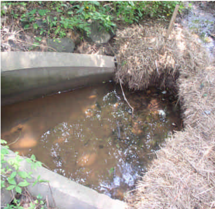
Haybales remain staked in place for additional filtration at the storm drain outlet. Water from the outlet was clear.
