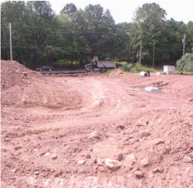
New site entrance to be constructed in this location with existing catch basin.
