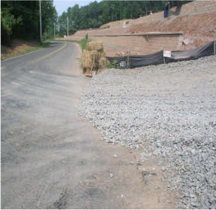
Crushed stone construction entrance pad is clean; loose stone continues to be pulled back off Carpenter Lane and the road should continue to be cleaned/swept, including the gutters by hand if necessary.
