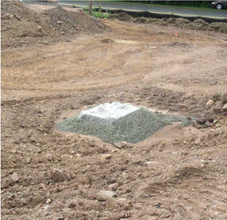
Catch basin inlet onsite is surrounded by stone and covered with fabric.
