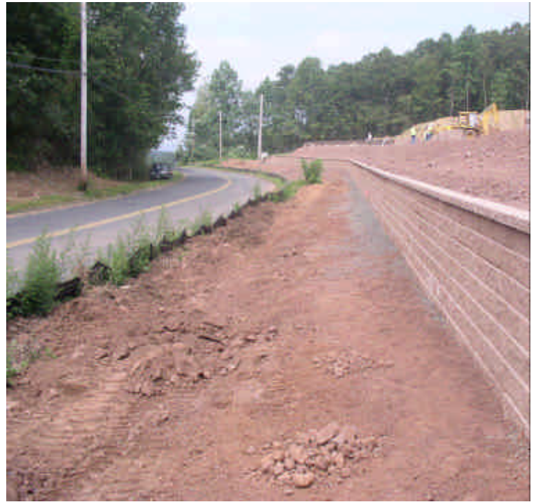
Grading and seeding remain to be done between Carpenter Lane and 1 st retaining wall.
