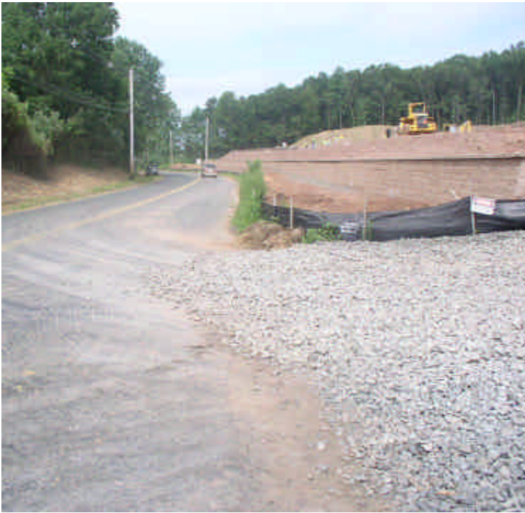
Crushed stone construction entrance pad is clean; loose stone should be pulled back off Carpenter Lane and the road cleaned/swept, including the gutters by hand if necessary.
