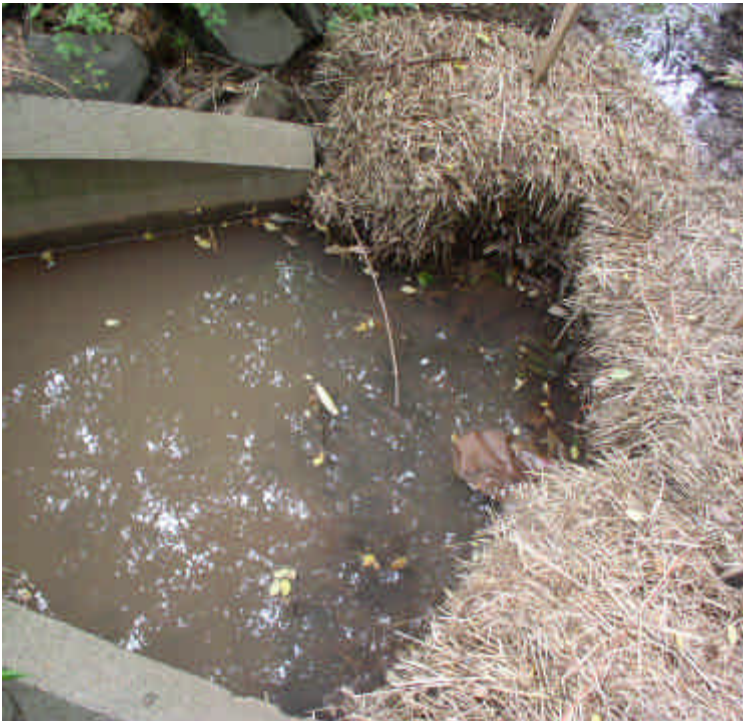
Haybales remain in place for additional filtration at the storm drain outlet. Water from the outlet was slightly turbid.
