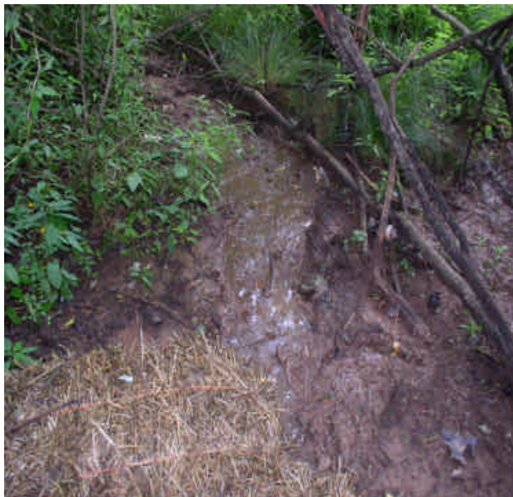
Water filtering through the haybales had improved clarity. Sediment accumulation from the previous rain events will be removed when conditions have dried out.
