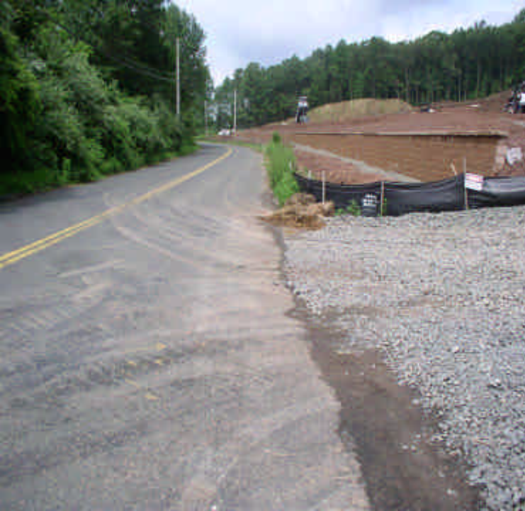
Crushed stone construction entrance pad is still clean, with some minor sediment tracking visible on Carpenter Lane.
