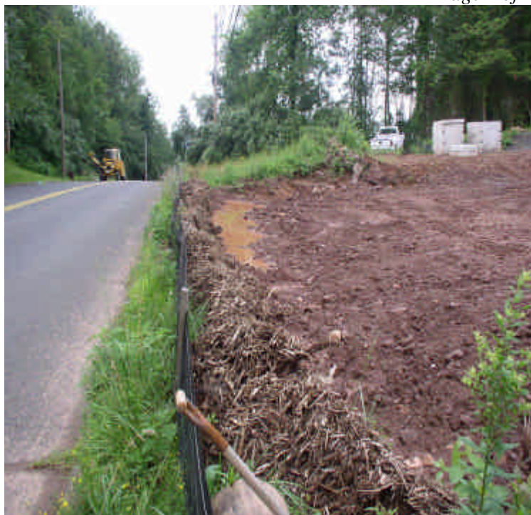
New water settling area dug in the southwest corner of the site.
