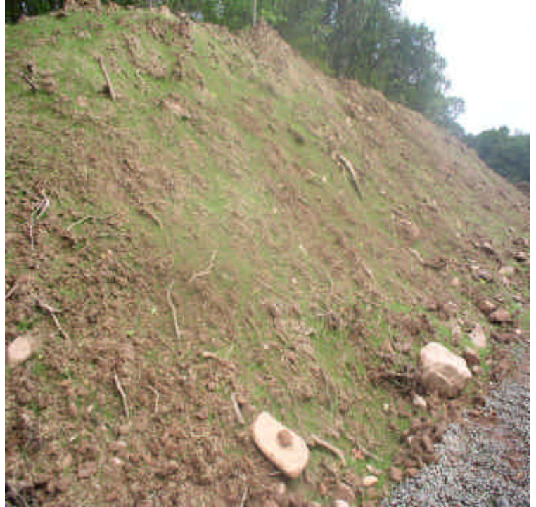
Grass growing on the newly seeded soil stockpiles.
