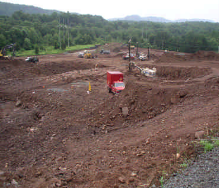
Entire site from northwest corner looking southeast at major grading and blasting operations.
