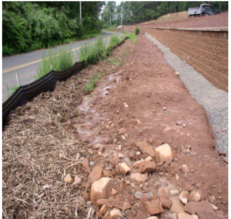
Bark mulch and silt fence along Carpenter Lane and new stone wall. Stormwater is being diverted to a settling area onsite.
