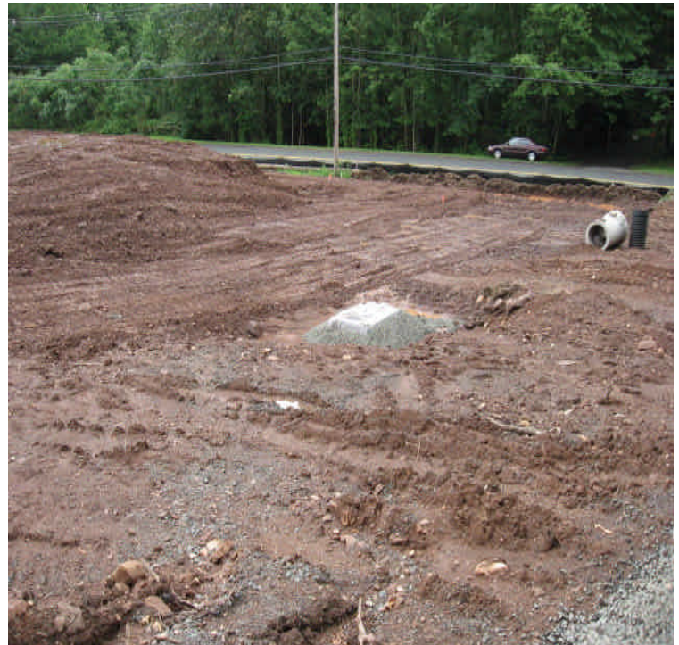
Raised catch basin onsite, surrounded by stone and covered with filter fabric.
