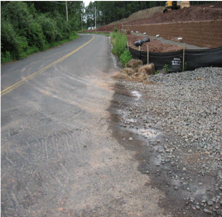
Crushed stone construction entrance pad is still clean, with some minor sediment visible on Carpenter Lane.
