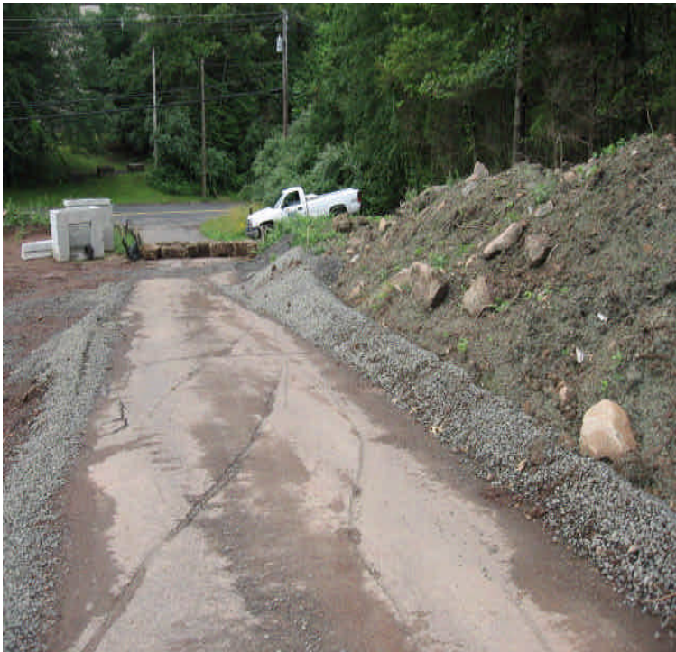
Haybales across old Zolnik driveway; soil stockpile to right has been hydroseeded and stone berm installed to filter runoff.
