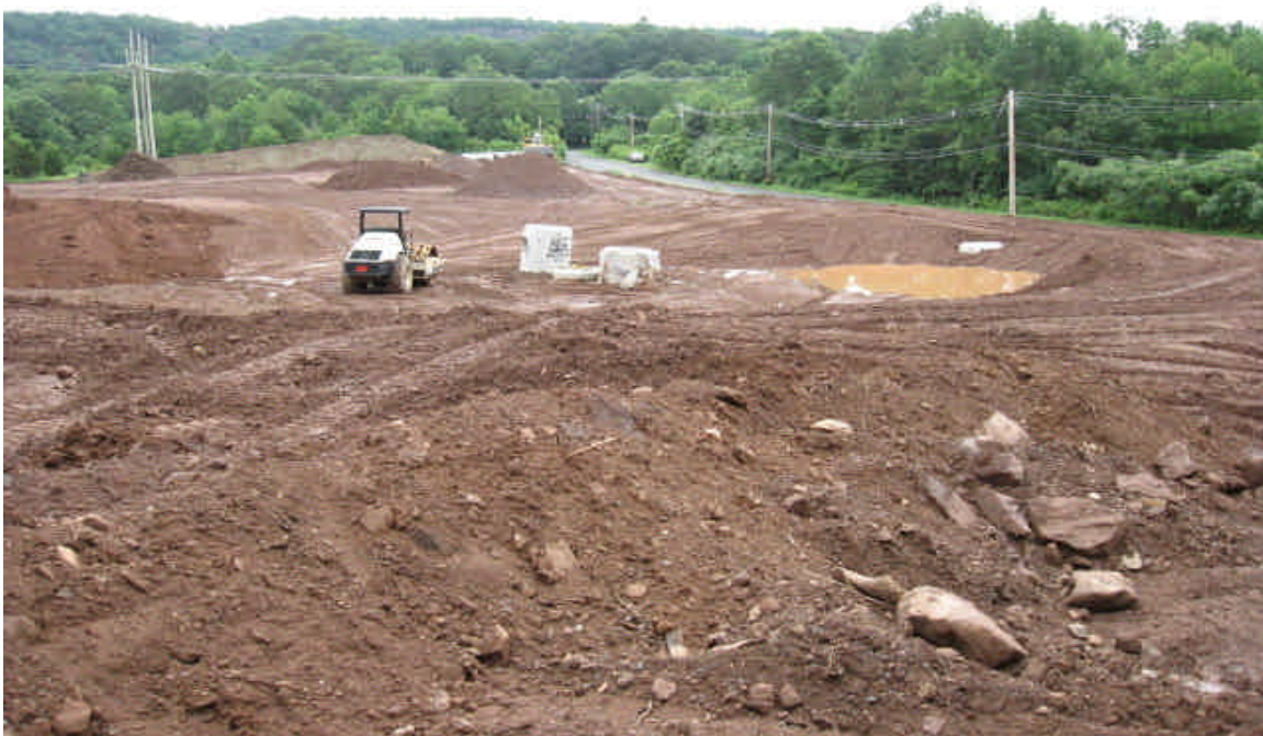
Temporary settling basin has been excavated north of the drain inlet pipe. However, it appears that the majority of turbid water to the wetland across Carpenter Lane may be coming from site run-off to the roadway catch basins
