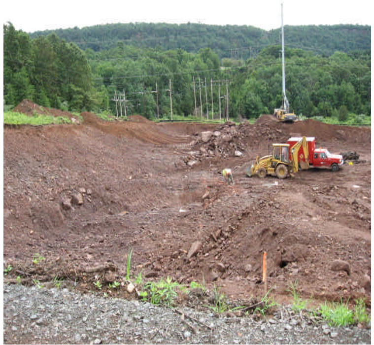
Preparations are being made for continued blasting on the northern portion of site.
