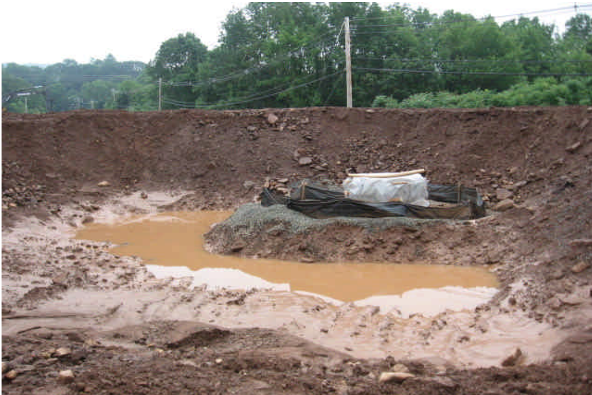
Temporary settling basin has been excavated around protected drain inlet pipe. However, sediment from site continues to enter wetland across Carpenter Lane.
