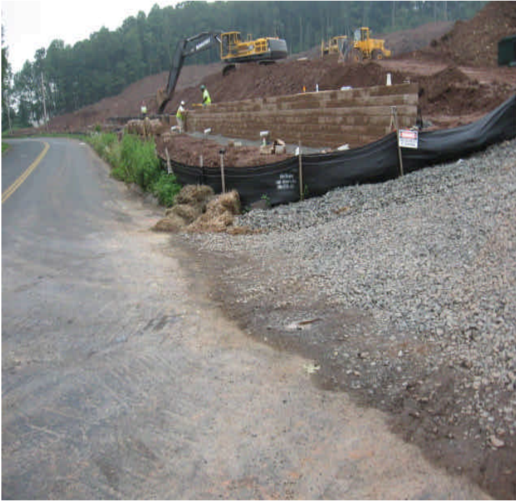
Crushed stone construction entrance pad is still clean, and only a minimal amount of soil is visible on the road.
