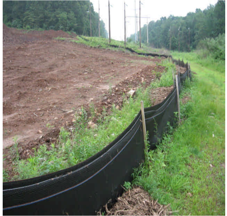
Silt fence on east side is reinforced with bark mulch. Buffers of vegetation also remain on both sides of silt fence, protecting wetland east of site.
