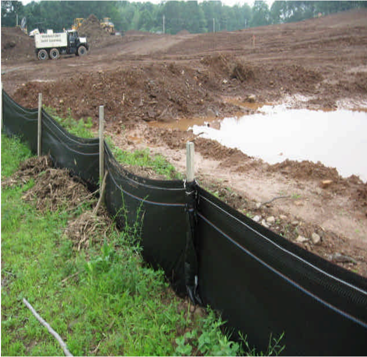
Stormwater has accumulated inside the silt fence near east side of site; no evidence of damage or stress to silt fence.
