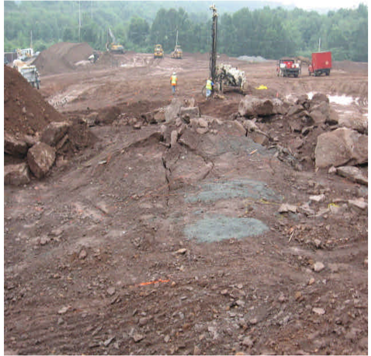
Preparations are being made for continued blasting on the northern portion of site.
