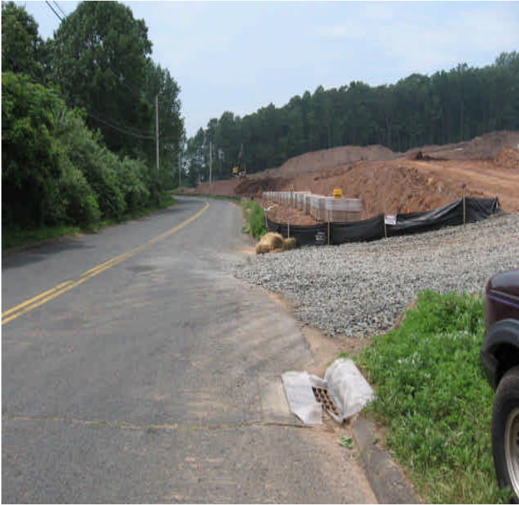
Negligible amount of soil visible on Carpenter Lane.
