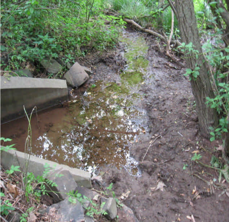
Drain outlet in wetland with clear standing water, accumulated sediment.
