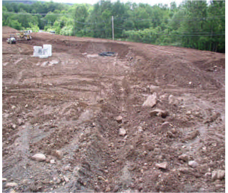
Construction is underway on the new retention ponds and storm water system along Carpenter Lane. Note the new drainage ditch installed to prevent run-off from bypassing the storm water system.
