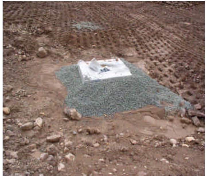
New CB installed along the southwestern side of the site is elevated, surrounded with stone, and covered with filter fabric to allow settling and filtering of storm water before it enters the CB.
