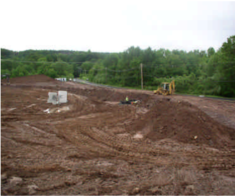
Construction is underway of the new retention ponds and storm water system along Carpenter Lane
