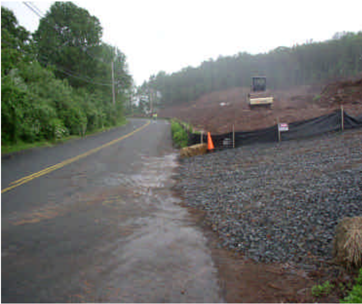
Carpenter Lane at the construction entrance. Entrance is clean and workers were replacing the filter fabric in the catch basins.
