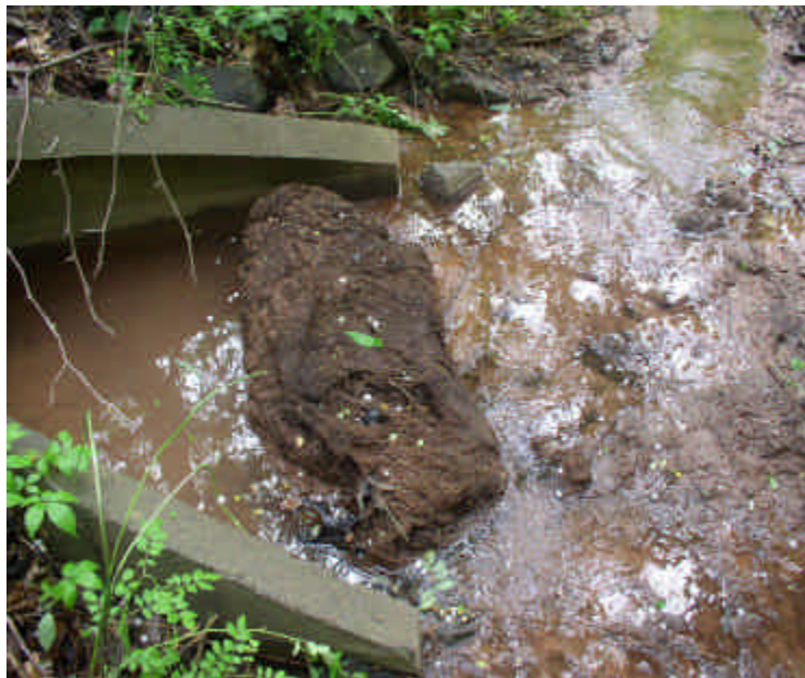
Storm water entering the wetland across Carpenter Lane is turbid, due to the interim of the installation of the new drain system on site and heavy rains. A large root ball has made its way through the system and is slowing water. Consider placing haybales here for further filtration.
