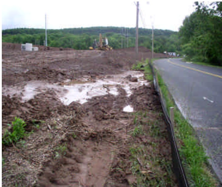
Temporary storm water settling area constructed to prevent runoff onto Carpenter Lane. This area is full of sediment and may need to be enlarged to keep stormwater contained to site.
