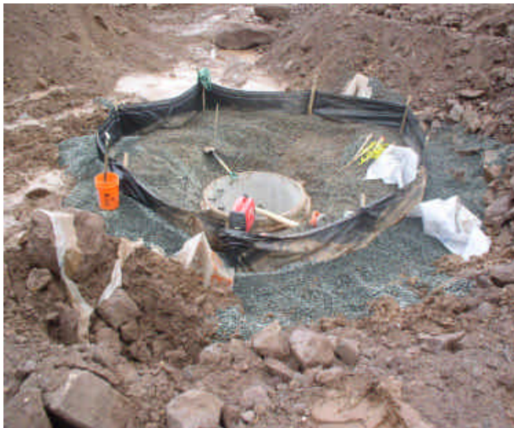
Installation of the new storm drain system. With perimeter protection. Watch exposed soil around the pipe for run-off and increase controls around the pipe.
