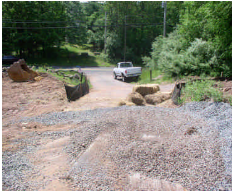
Haybales will be replaced across the western driveway where they were moved to dump stone for the installation of the new storm water system. Watch potential run-off here.
