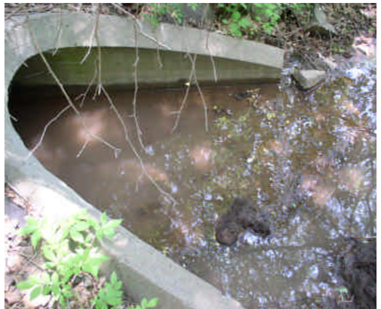
Storm water entering the wetland across Carpenter Lane is slightly turbid, resulting from the installation of the new drain system on site. This will be difficult to control until the new system is in place.
