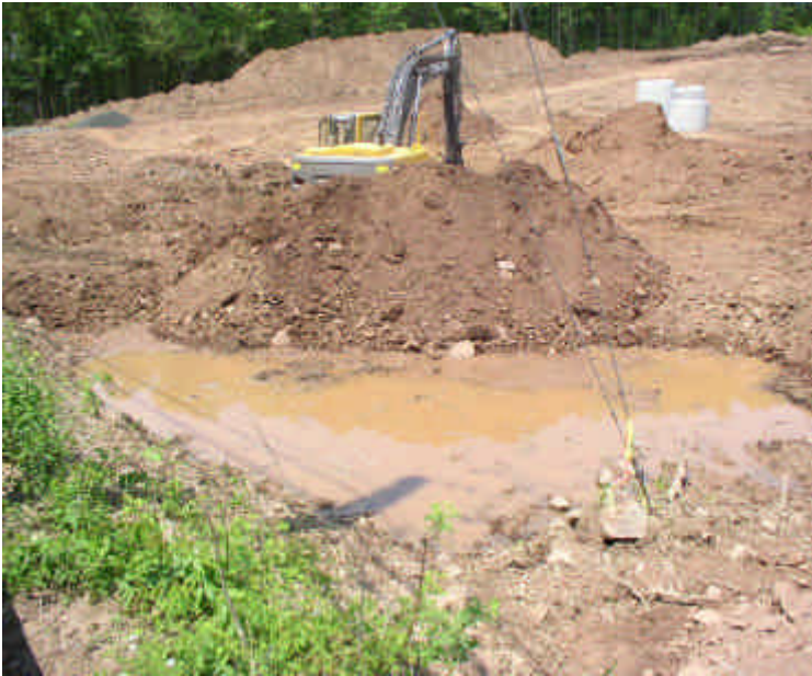
The old settling basin has been partially filled and closed off to the new storm drain. Saturated soil is being piled here from the adjacent excavation.
