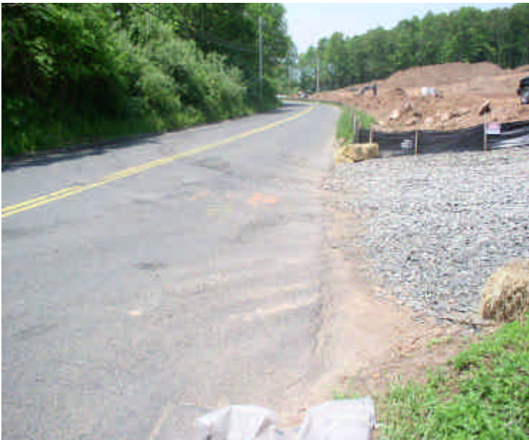
Carpenter Lane at the construction entrance, where tracking into the warm roadway pavement was noted. Small stones were swept up immediately.
