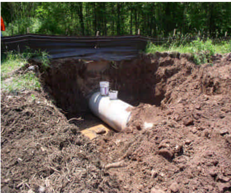
New storm drain outlet connection to the existing catch basin at Carpenter Lane.
