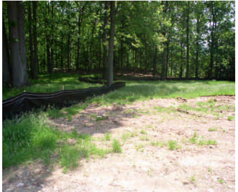
Silt fence installation is complete around the old Zolnik property. No soil is being stockpiled here yet.
