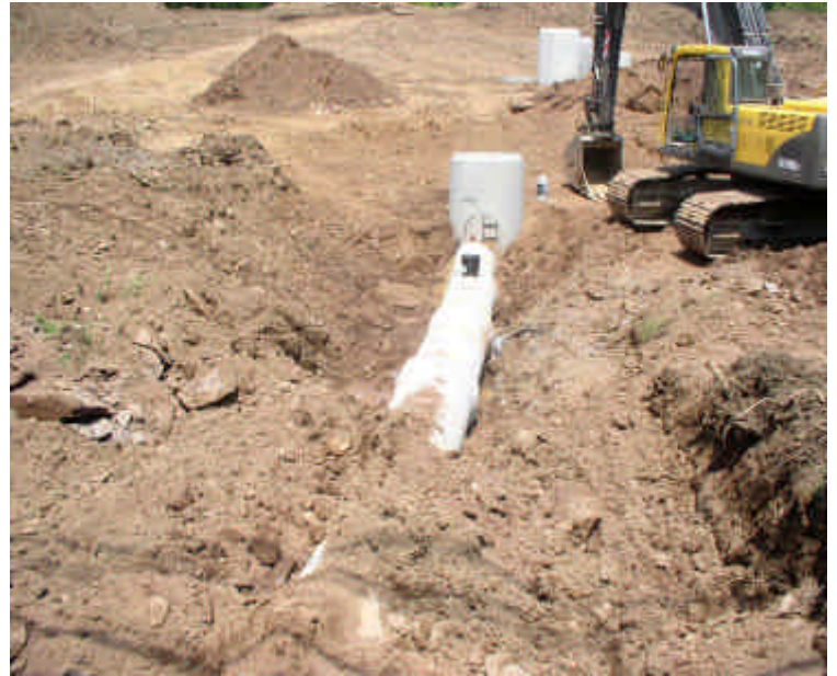
Installation of the new storm drain system. The drain pipe is being extended to a new catch basin.
