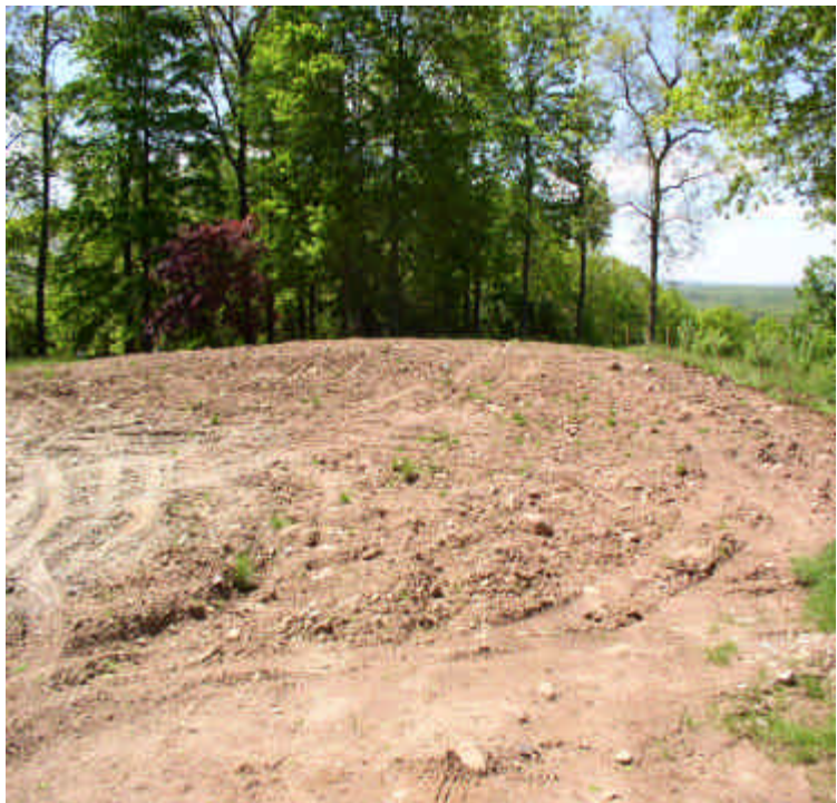
New soil stockpile area located at the old Zolnik property. Silt fence was being installed in this location
