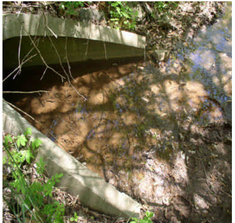
Storm water outlet to the wetland across Carpenter Lane. Water entering the wetland was clear at this time.
