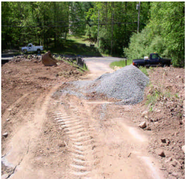
Haybales will be replaced across the western driveway where they were moved for access to the new stockpile area.
