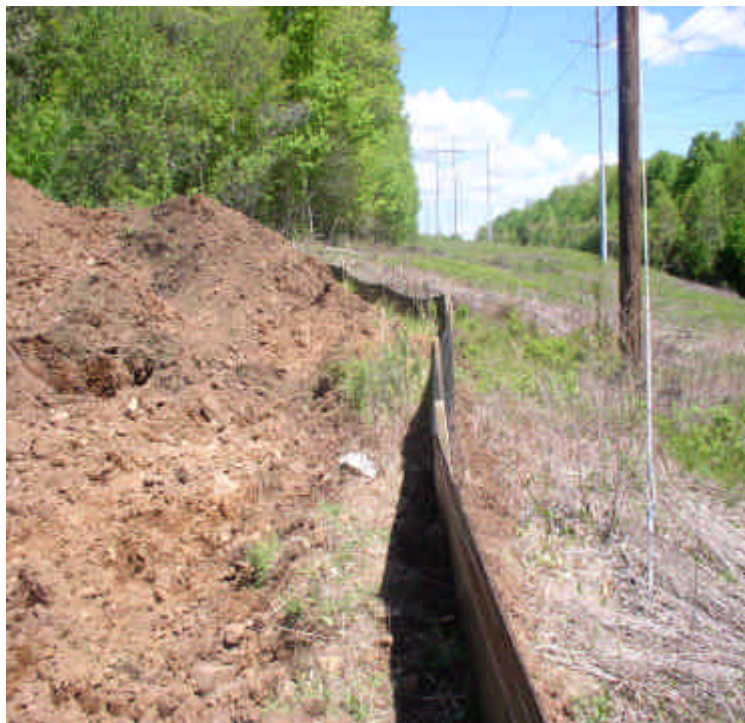
New silt fence was extended along the northeast corner of the site to encompass the work limits.
