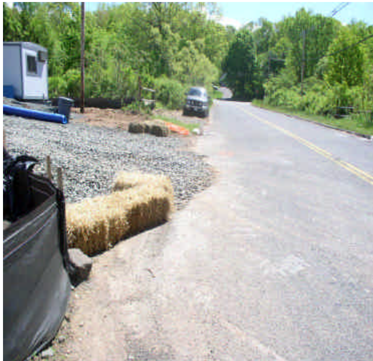
Carpenter Lane at the construction entrance. No significant sediment tracking was noted.
