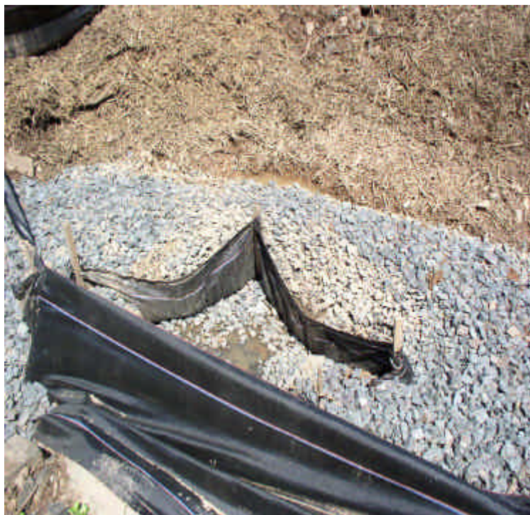
Storm drain inlet leading to wetland across Carpenter Lane. Even though a number of additional controls have been placed, water remains turbid leaving site.
