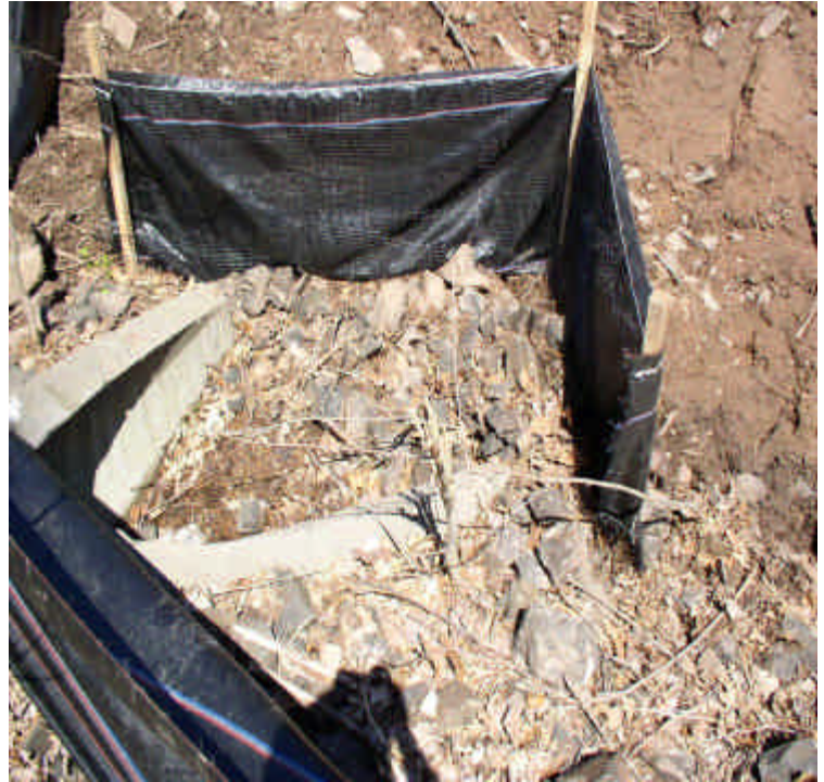
Storm drain inlet (leading to wetland across Carpenter Lane), with secondary silt fence and riprap in place.
