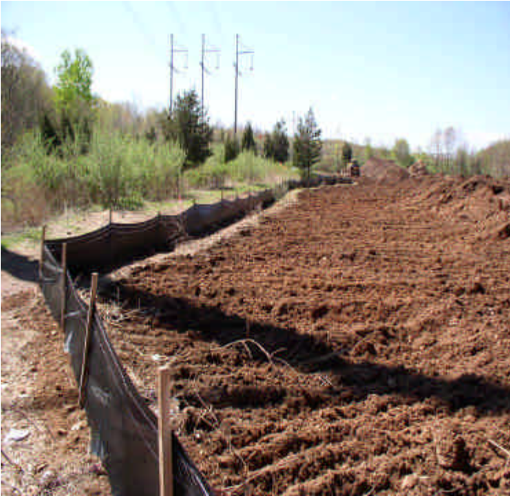
Silt fence installation is complete around the eastern and western work limit lines.
