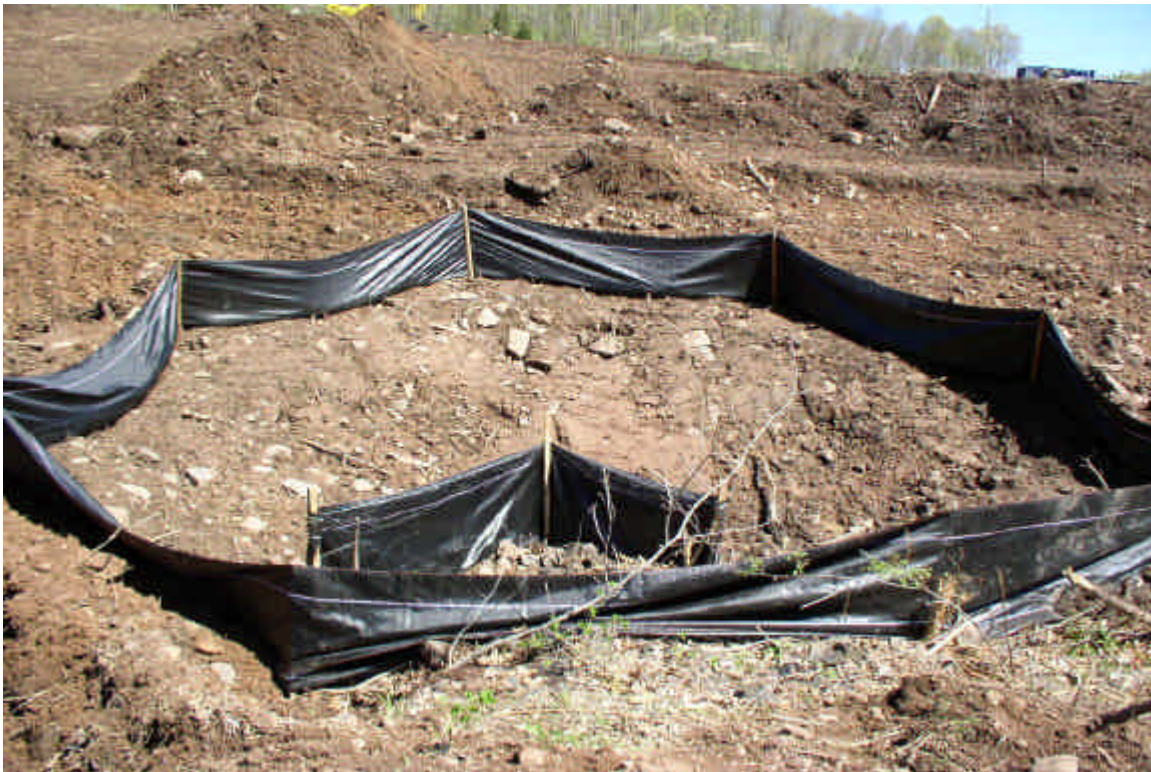
Additional silt fence was installed around the storm drain inlet. Consider providing stabilization measures within the enclosure to further reduce potential sedimentation.
