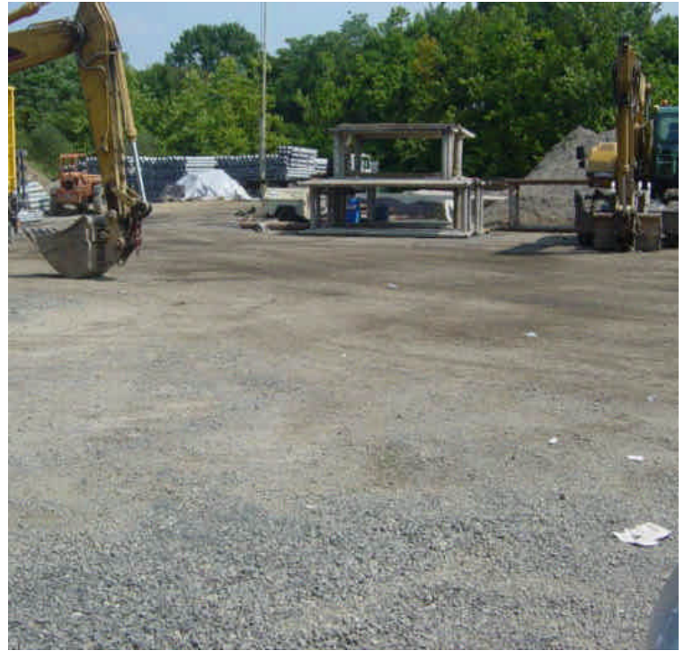
Calcium chloride has been spread throughout the King's Highway laydown yard to aid in reducing airborne dust generation.
