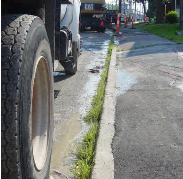
Dust/slurry was observed along on the edge of the roadway from recent sawcutting activities near sta. # 775. Continue to attend to cleaning up this material as soon as it is generated.
