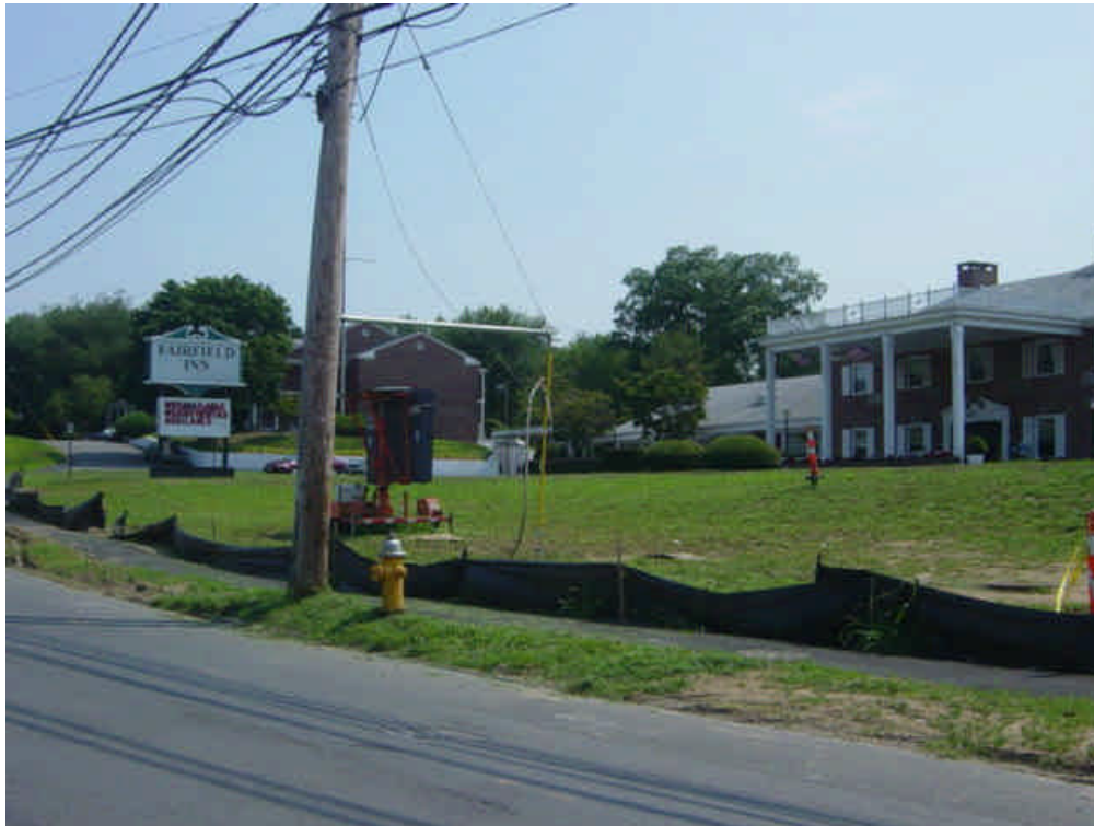
Erosion controls are in disrepair near vault #37. Either maintain the controls or remove them if the adjacent area is fully stabilized.
