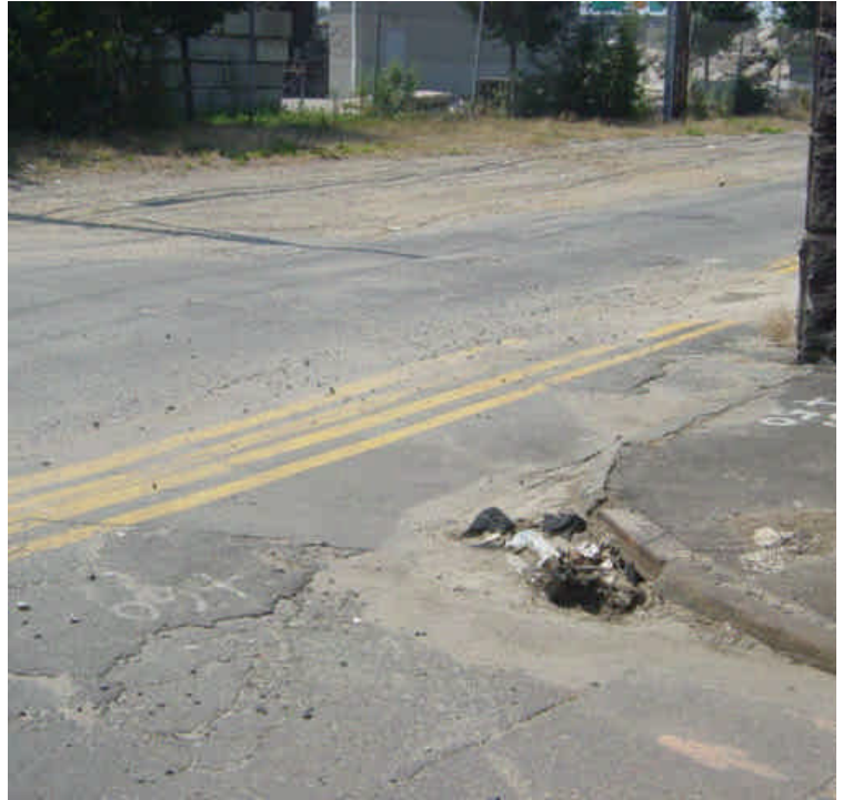
Catch basins located at the intersection of Railroad Ave. and Hancock Ave. are overwhelmed by sediment and debris. Some of the material appears to be from deteriorating patches or fill covering the trench.
