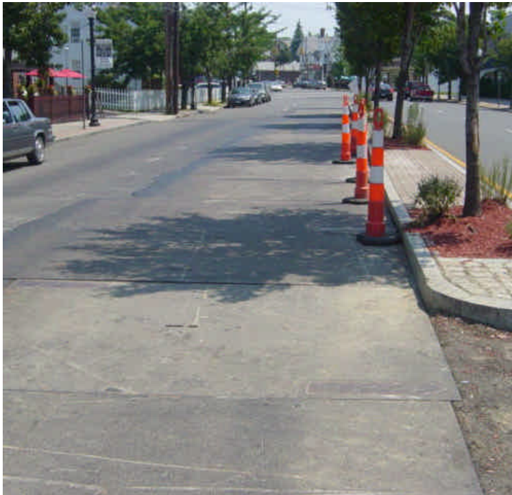
Photo of a typical active area of construction as it looks during the daytime, with trench covers in place.
