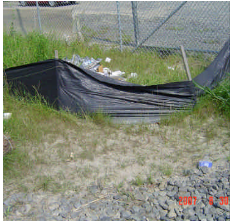
Non-project related debris was noted dumped just outside the entrance to the Milford yard. Although this is not the contractors' responsibility, consider disposing of it for appearances/aesthetics.
