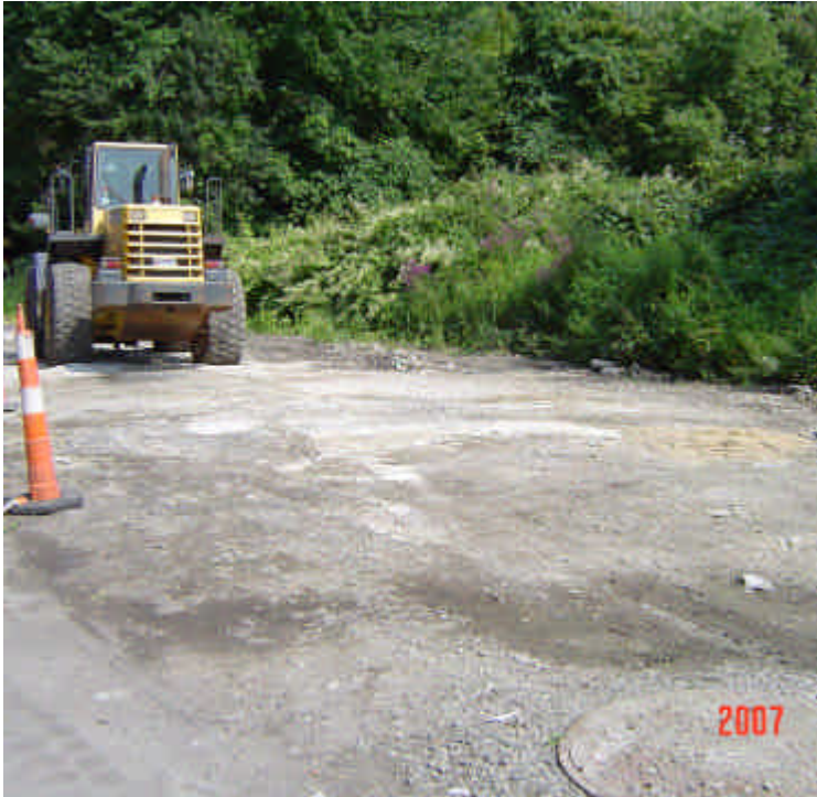
View of the area near Vault #1. Construction activities that are not part of the Middletown/Norwalk continue here and impede any further stabilization efforts. These contractors also continue to have washouts here.
