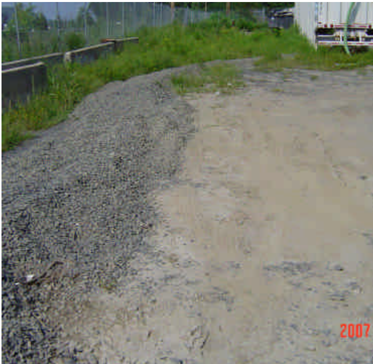
The stone berm remains in place at the Milford lay-down yard and continues to prevent sedimentation outside of the yard.
