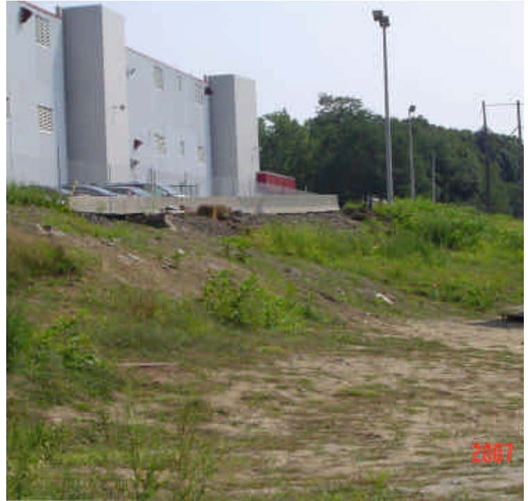
View of the slope near Sta #1080 which is partially stabilized. Contractors are going to work out a final stabilization plan in the future.
