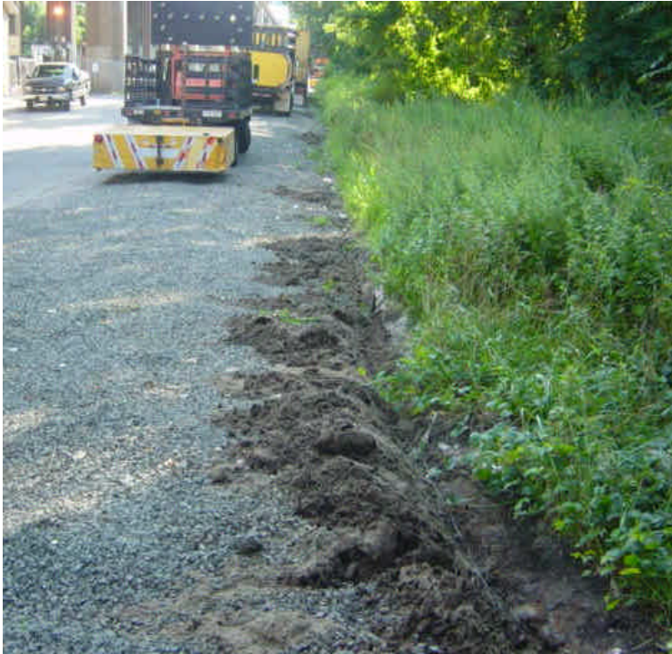
Silt fence has been removed near sta. # 1017 as adjacent areas are stable. It would be beneficial to apply seed to the areas exposed by the removal of the fence.
