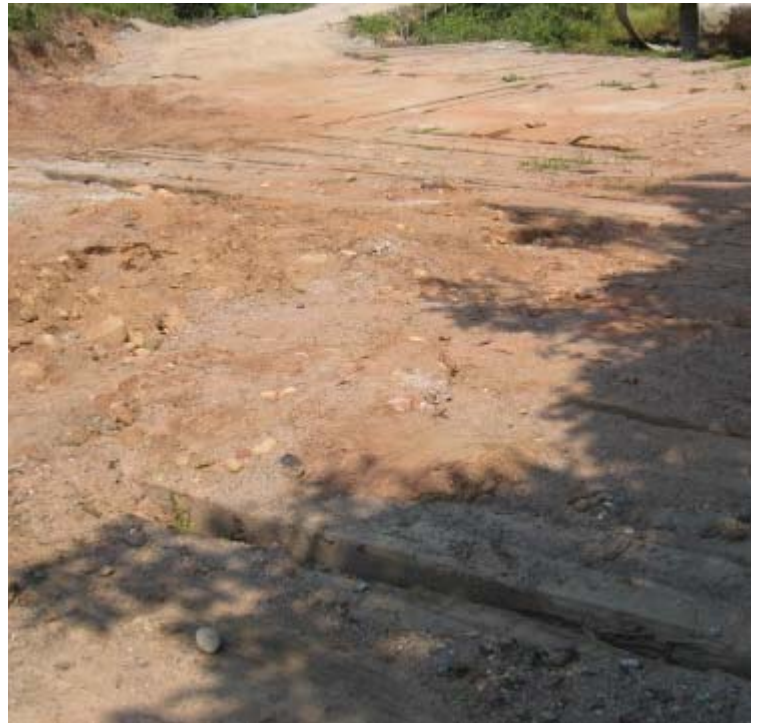
Willow St: Excess soil remains on the Timber Mats at structure #4009.
