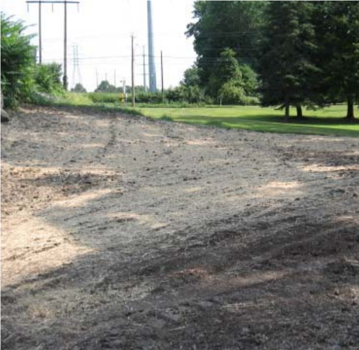
Wheelers Farms Rd (Milford): Exposed soils from pad reclamation activities have been temporarily stabilized with mulch.
