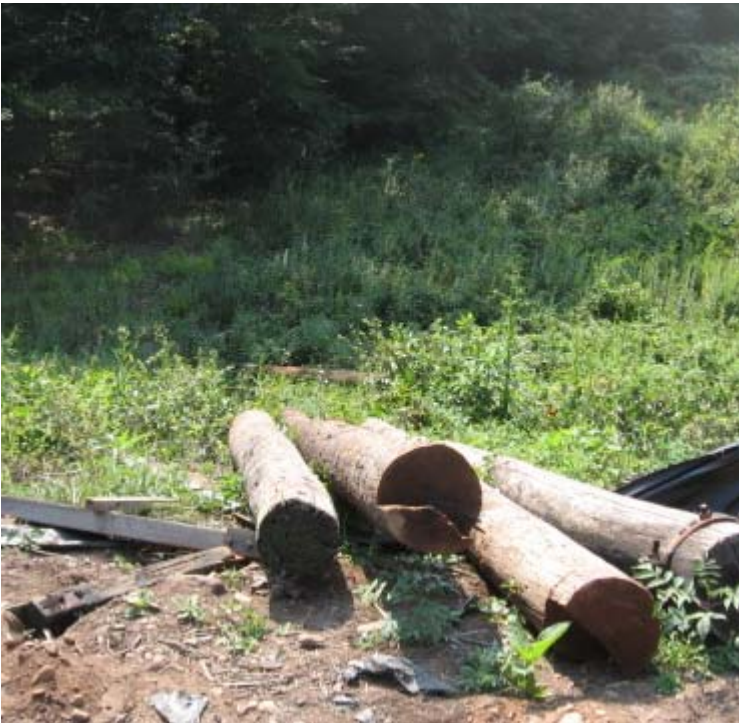
Willow St. (Hamden): Disassembled H-frame structures were noted on top of the silt fence and in a wetland buffer near structure #4010.
