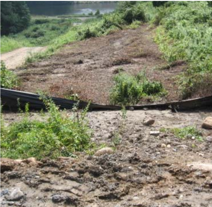
Glen Dam: Silt fence is in need of repair here and soils remain exposed adjacent to structure #3950.
