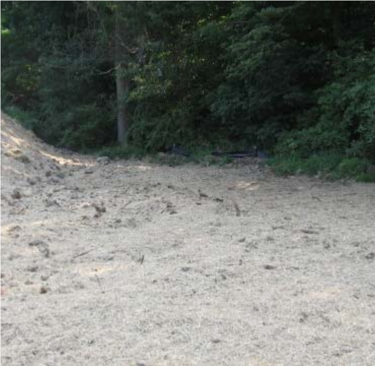
Lexington Lane (Milford): Rock has been pulled away from the silt fence as part of the pad reclamation work. Exposed soils have been mulched.
