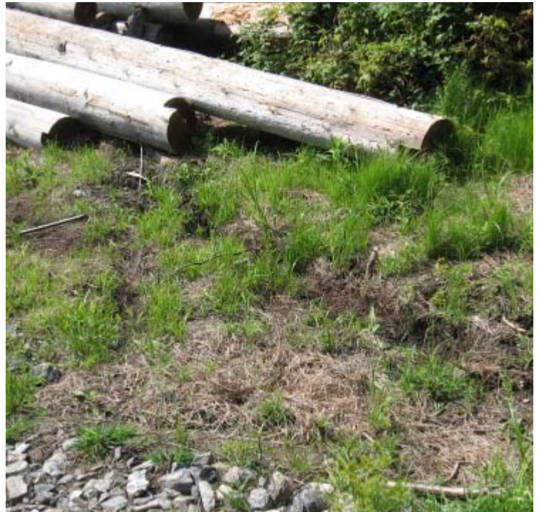
Hatfield Rd (Bethany): Ruts from foundation work and a disassembled H-frame structure remain in the wetland here.
