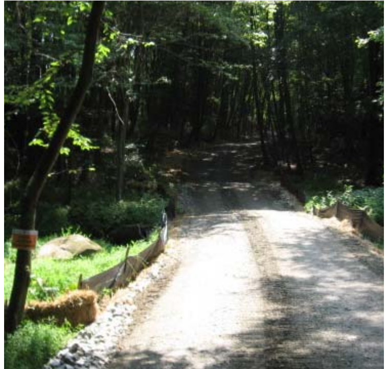
Clearview Ln. to Rte. 15 (Woodbridge): A view of the access road at the stream crossing. Proper controls are in place.
