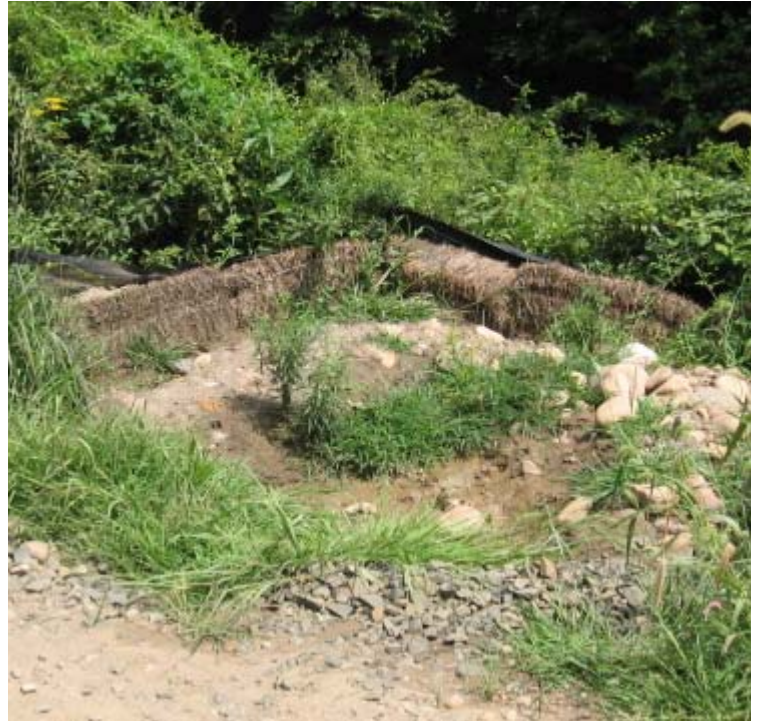
Glen Dam (Woodbridge): Sediment has accumulated in the stone lined sediment trap here.
