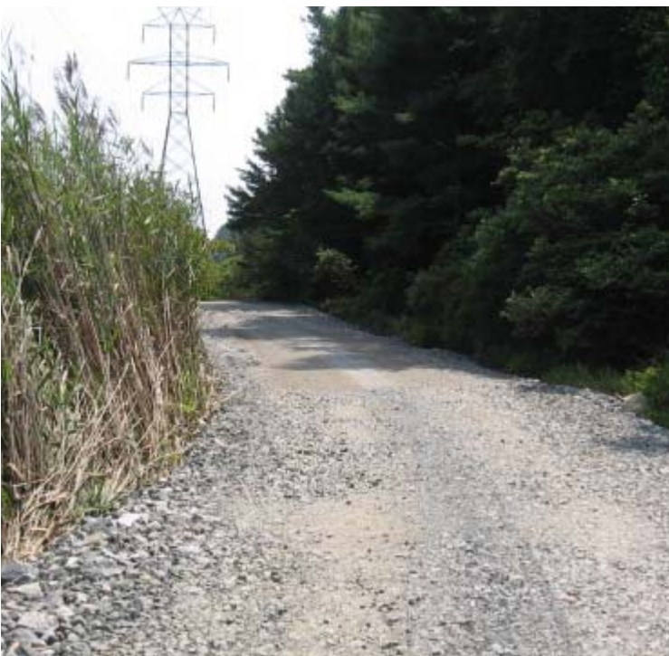
Clearview Ln. to Rte. 15: A view of access road construction through the wetland near structure #3899.
