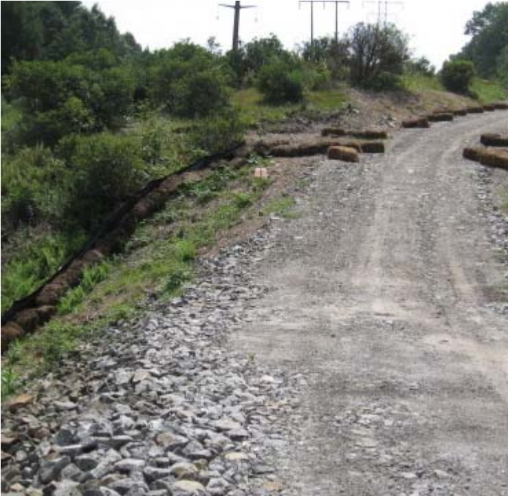
Litchfield Turnpike (Bethany): Haybale check dams have been added along the access road where washouts have occurred in the past.
