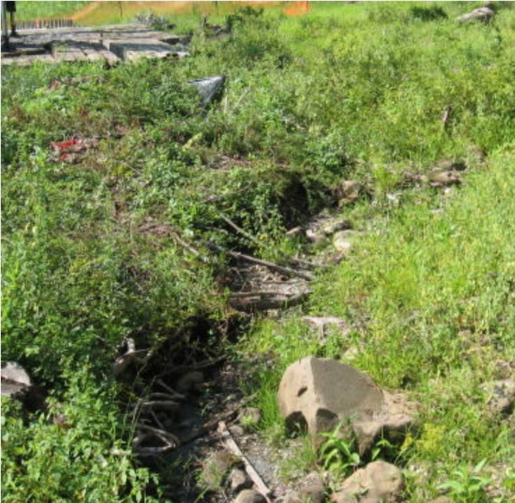
JCC (Woodbridge): The silt fence is in need of repair near proposed structure #24119. Also, sediment from foundation work was noted in the dry stream channel.
