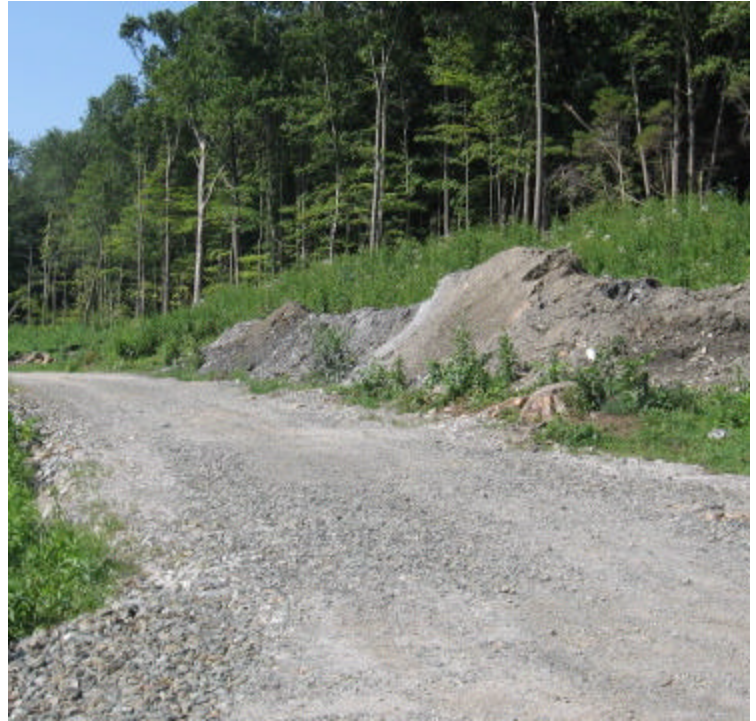
JCC (Woodbridge): Uncontained spoil piles were noted upgradient from the wetland here.
