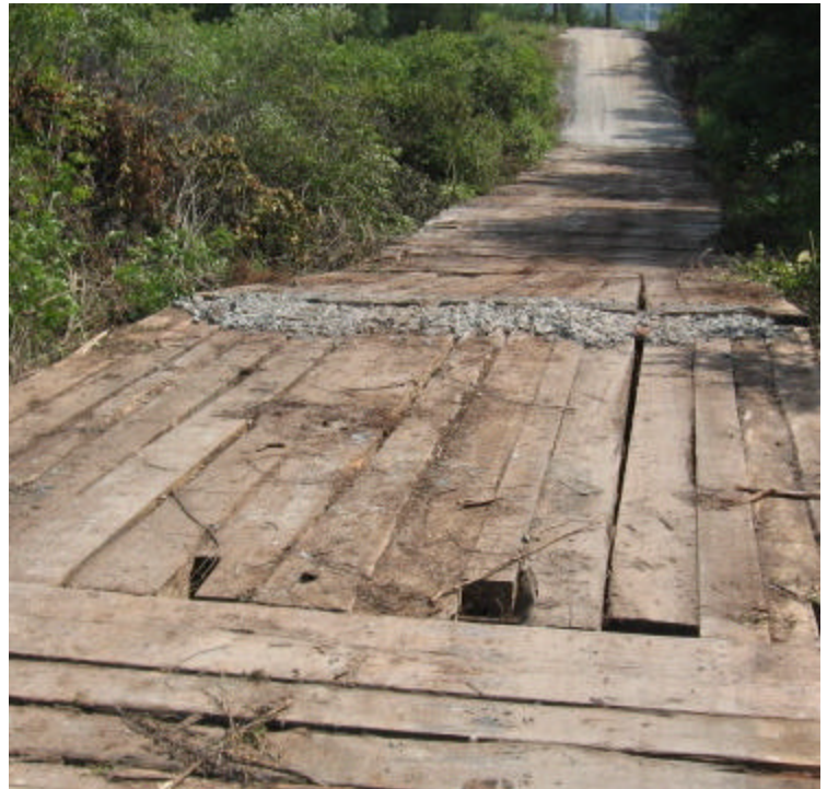
Brooksvale east (Hamden): Timber mats have been installed at the wetland crossing here.
