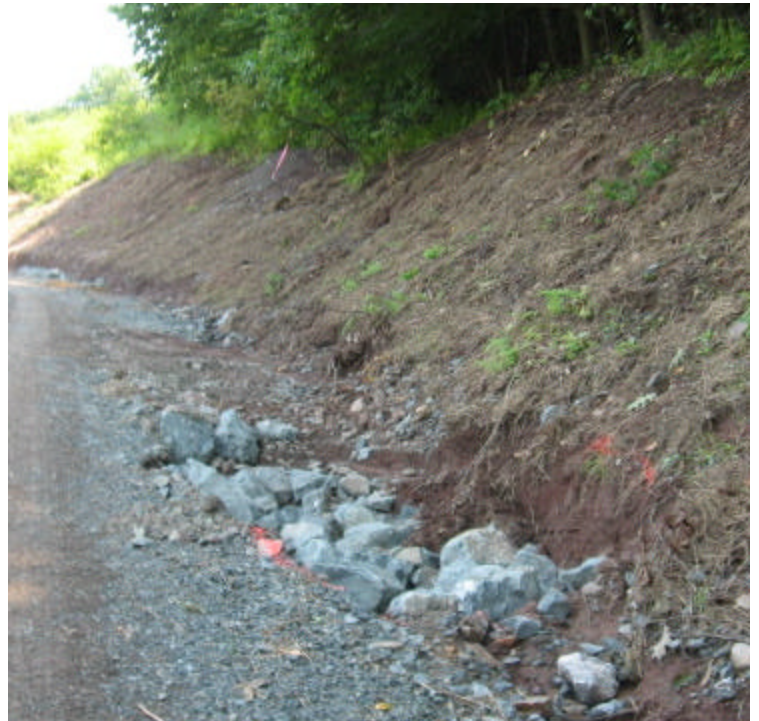
Old Lane Rd (Hamden): Washouts have been stabilized with stone, but some sediment remains within the wetland here.
