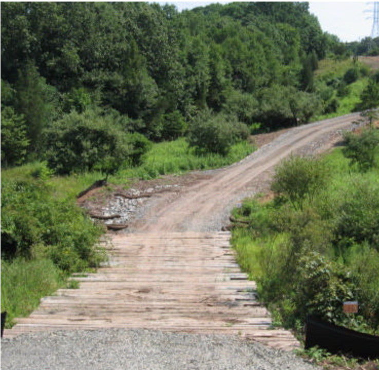
Brooksvale west: Timber mats are in place at the second wetland crossing. Silt fence is in place and controls will continue to be added as work progresses.
