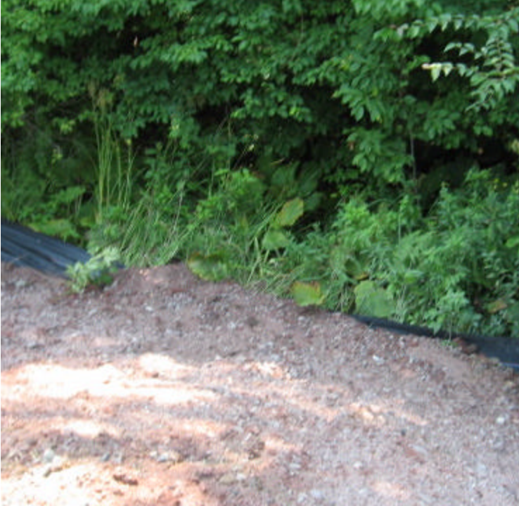
West Todd NE (Hamden): Spoils from foundation work have overwhelmed the silt fence and are now in the wetland here.
