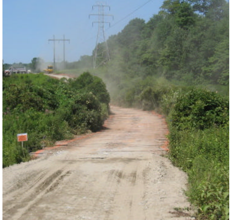
Brooksvale west (Hamden): Timber mats are in place at the wetland crossings. Erosion controls are being installed as work progresses. Dust control was not provided on site.
