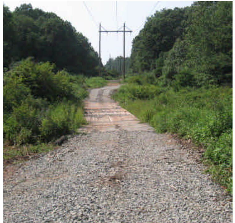
Pond Hill Rd: View of the timber mats in place at the wetland crossing.
