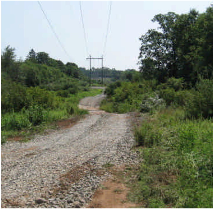
Pond Hill Rd: A view of the access road being installed here.
