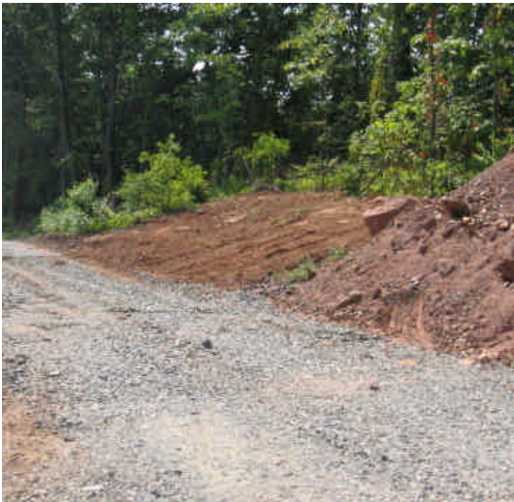
Williams Rd: Exposed soils remain near a wetland after access road construction. Seed the slopes or temporarily stabilize to prevent run-off.
