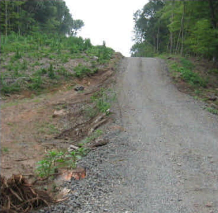
Ruts/washouts have been regraded along a steep slope in the access road off Black Walnut Drive.
