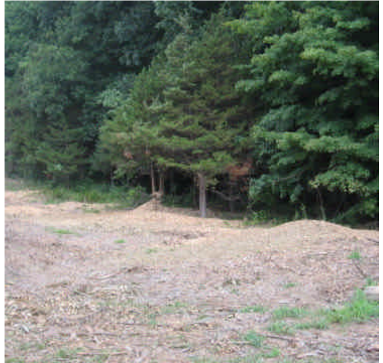
Black Walnut Dr: Wood chip piles, greater than three inches deep remain in the ROW at the 1A/1B intersection. Spread chips out in upland areas or remove from the ROW.
