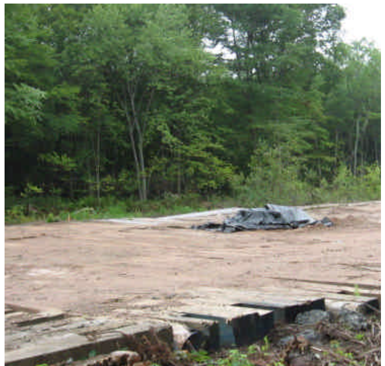
Some accumulated sediment remains on the timber mat crane pad west of Route 17. Remove if feasible to avoid run-off to the wetland
