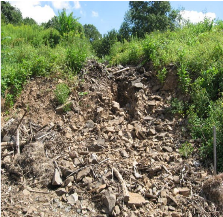
East Meriden SS: Run-off from substation is eroding the slope here.
