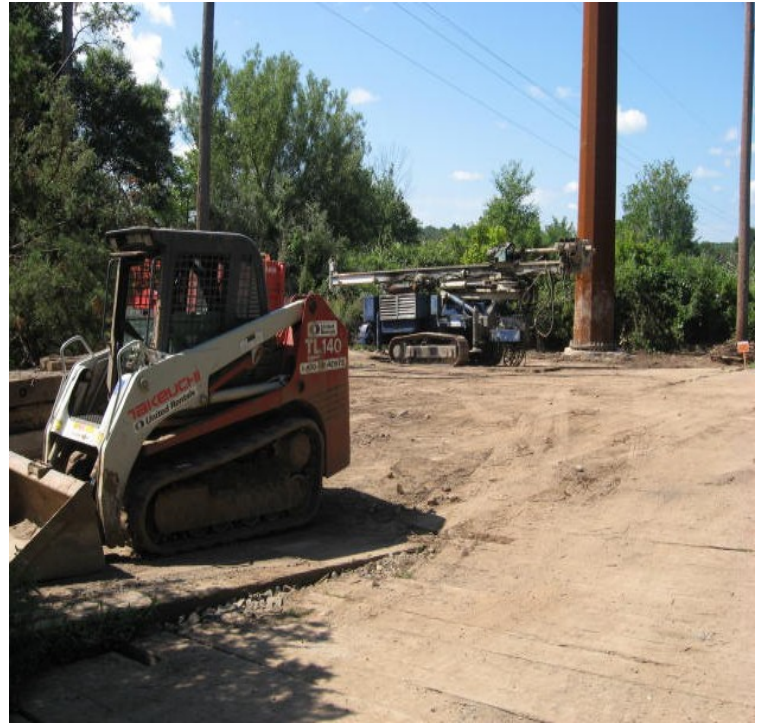
Durham Rd: Equipment stored within the wetland area.
