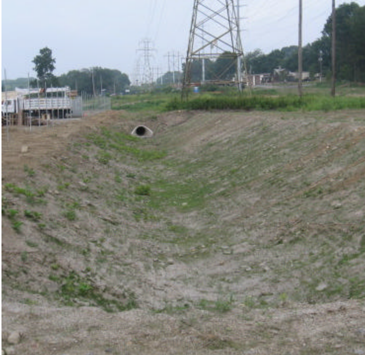
Grass growth was noted in the drainage swale.
