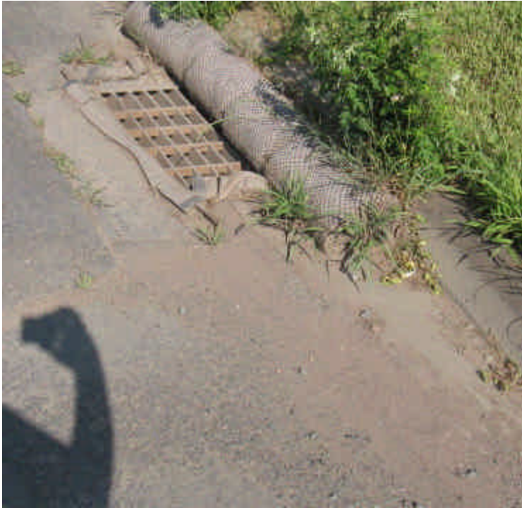
Some sediment accumulation remains around the catch basins along Carpenter Rd.
