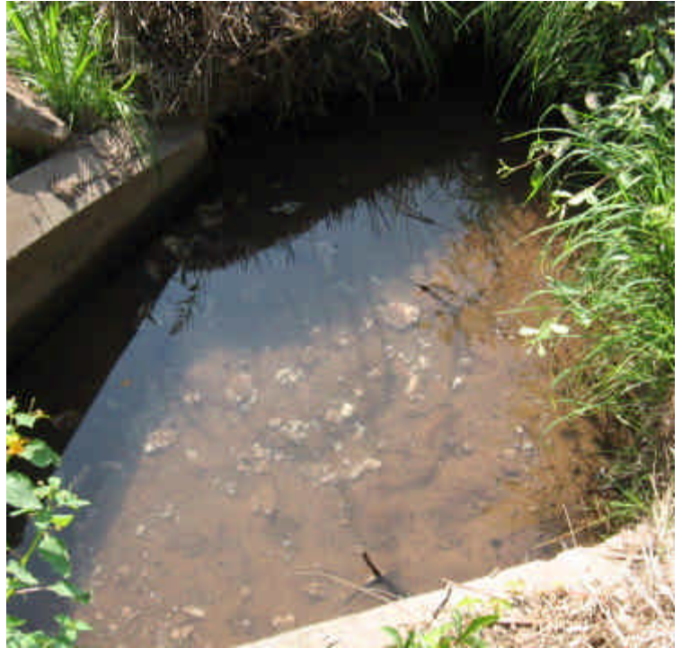
Sediment has settled out of the standing water and accumulated at the culvert outlet south of Carpenter Rd.
