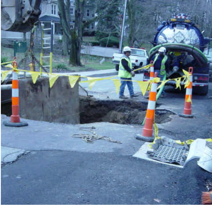
Construction activities located within Imperial Ave. adjacent to Dead Man's Creek. Adjacent catch basins have been protected.
