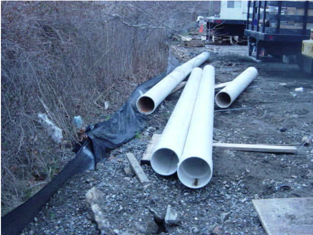
Materials within the King's Highway lay-down yard were piled against the controls, compromising them. The fence should be re-established. Continue to store materials in a way that does not strain the controls.
