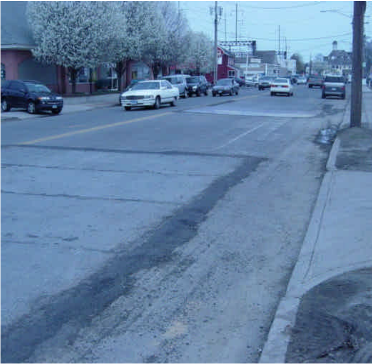
Photo of vault #32, minor sediment/material accumulation was noted along the shoulder of the roadway. Provide regular sweeping along the roadway, including the gutters.
