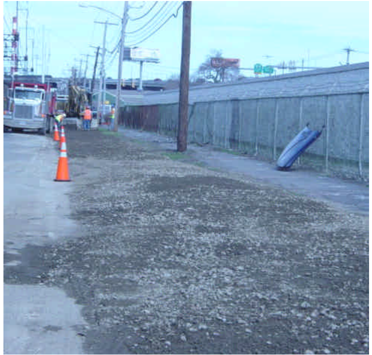
Stone is being applied to the ruts in the shoulder of Railroad Ave., and to prevent additional tracking.
