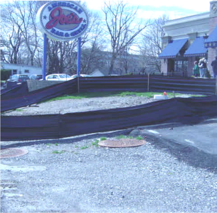
Well installation at vault #36 caused additional soil disturbance. Silt fence has not been toed-in, leaving it ineffective. The silt fence should be toed-in to provide the intended control.
