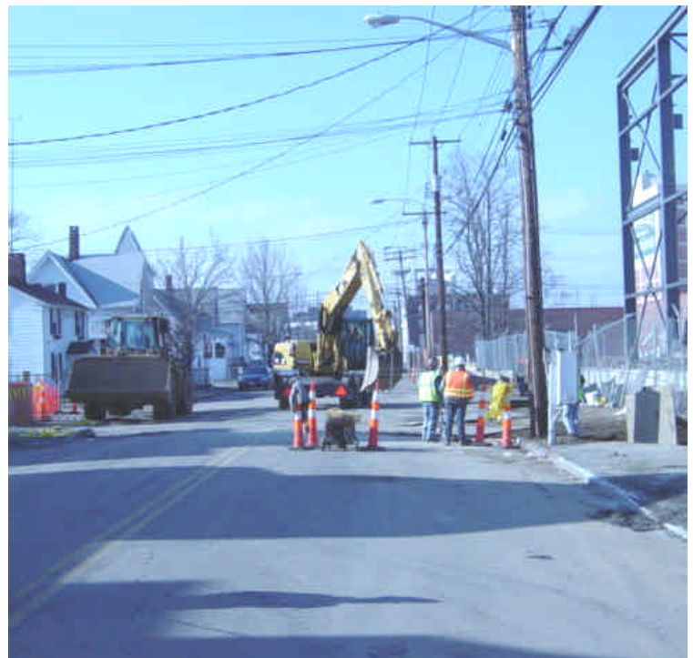
Trenching activities within Main St., located immediately adjacent to the fence at the Singer Substation yard. No issues were noted.
