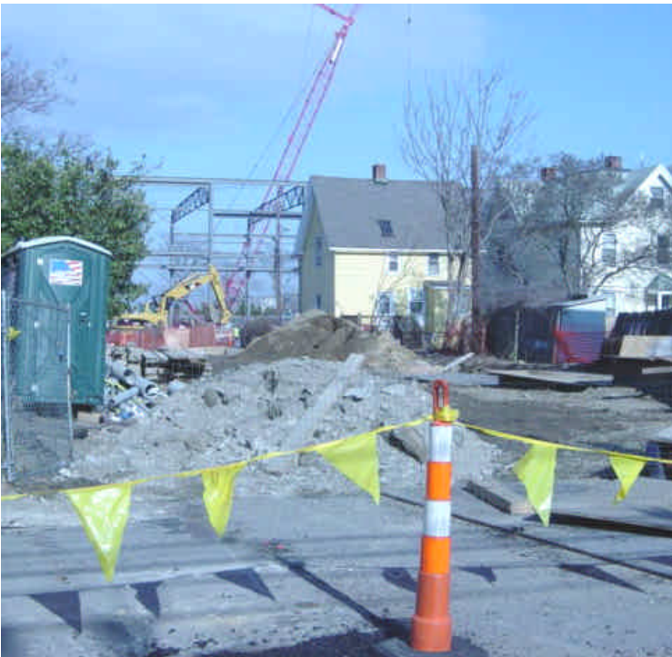
Photo of trenching activities between Broad St. and Main St. No issues were noted. Continue to keep soil contained to the work area.
